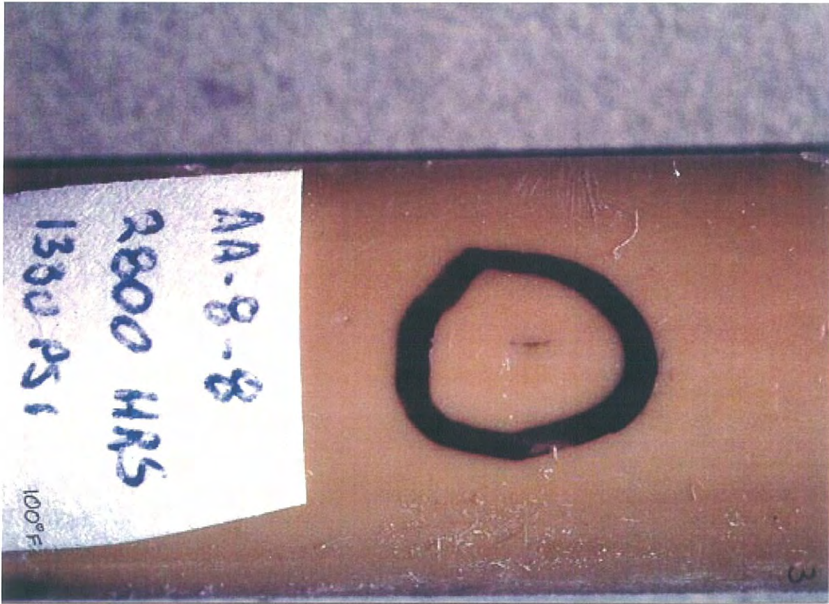
Figure 5 -- Slit fracture resulting from a stress rupture test conducted at 100 °F. Note lack of deformation visible in the fracture. This pipe was manufactured by DuPont in 1977. After failing Minnegasco's incoming inspection tests, the pipe was subjected to stress rupture testing. (Source: Henrich, R.C., and Funck, D.L., "Effects of ESCR Variation on Some Other Properties of Plastic Pipe." Proceedings, Eighth Annual Plastic Fuel Gas Pipe Symposium, 1983. )
