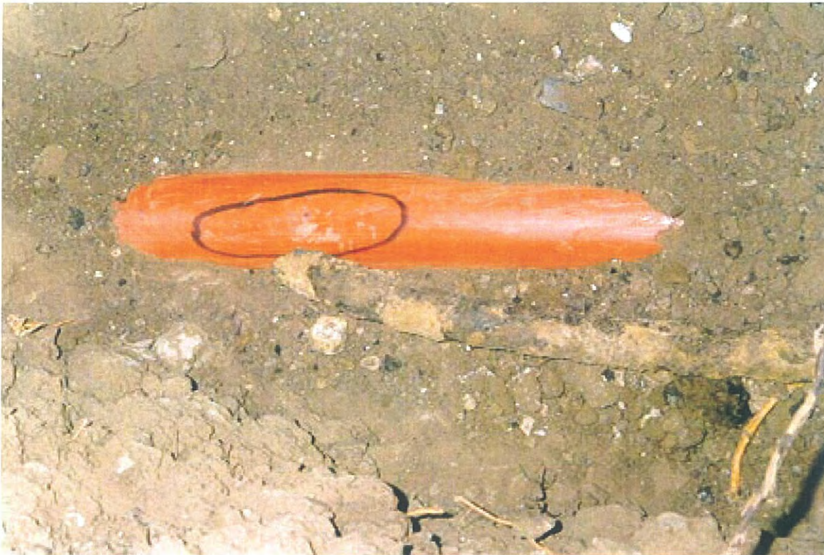
Figure 8 -- Brittle-like crack in pipe involved in August 1997 accident in Lake Dallas, Texas. The crack extends from the left to upper right of the area defined by the ellipse.
