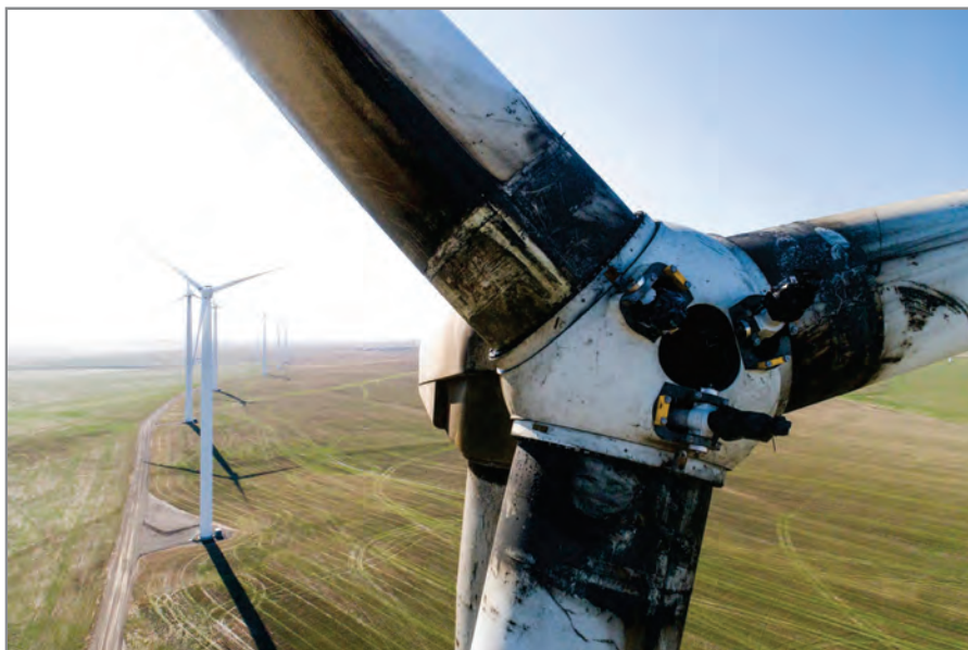
A metal frame and pieces of fiberglass fell from the spinner cone of this Vestas turbine into a field below at Biglow Canyon wind farm in April 2021. PGE didn't report the incident to regulators until this summer. Wind
