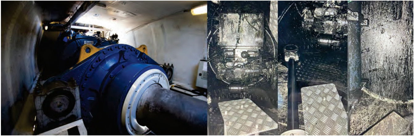
Portland General Electric provided a look inside the spotless nacelle of a Vestas turbines (left) at Biglow Canyon wind farm during a tour in late June. Kathryn McCullough sent the pictures at right to U.S. Sen. Ron Wyden, which she said shows the oil-coated nacelle of a Vestas turbine this spring at Biglow Canyon. (Photos courtesy PGE, left, and Courtesy Kathryn McCullough, right)
