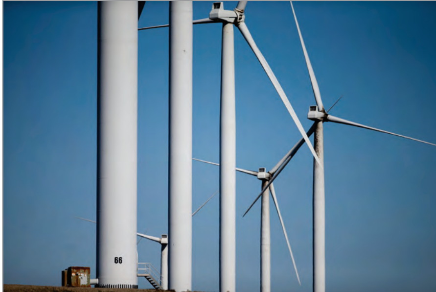
Residents who own land under PGE's Biglow Canyon wind farm worry that regular leaks of oil and lubricants from turbines pose fire and environmental hazards.
