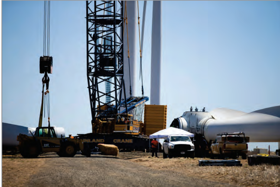
Workers replacing the blades on a Vestas V82 wind turbine at Portland General Electric's Biglow Canyon wind farm in late June. The turbine threw one of its blades into a wheat field on Feb. 1. PGE blamed "a loss of clamping force."
