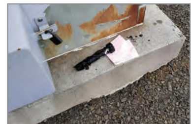
A broken blade bolt found under a wind turbine at Biglow Canyon wind farm by a worker delivering fertilizer in late January. A day or two later, the turbine threw an eight-ton blade into a nearby field. (Courtesy Kevin Massie)
