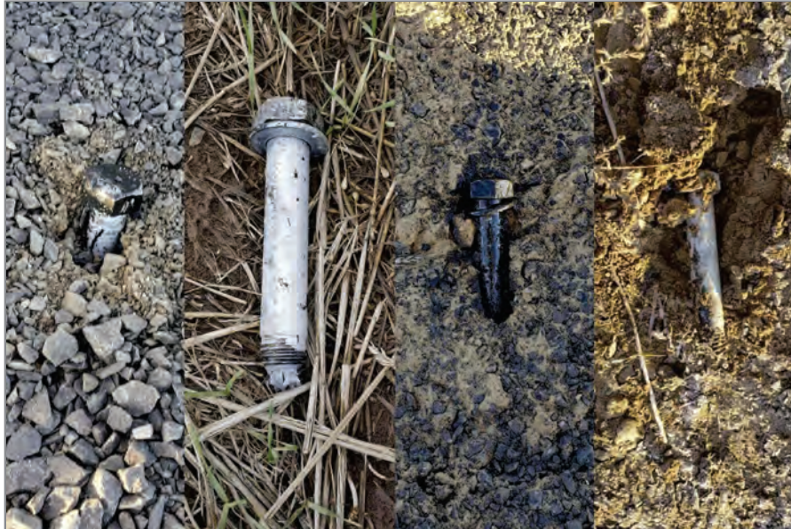
Broken blade bolts were scattered around turbine 71 at Portland General Electric's Biglow Canyon wind farm after the turbine threw a blade in the early hours of Feb. 1. Hours before the blade throw, a driver delivering fertilizer became stuck in close proximity to the turbine and had to be towed out. (Courtesy Kevin Massie)
