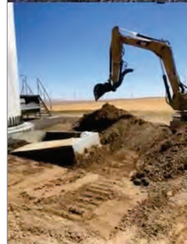
Screen shots of a ruptured transformer and the required cleanup of a transformer oil spill from a presentation that PGE made to state regulators in January about transformer problems at the wind farm.
