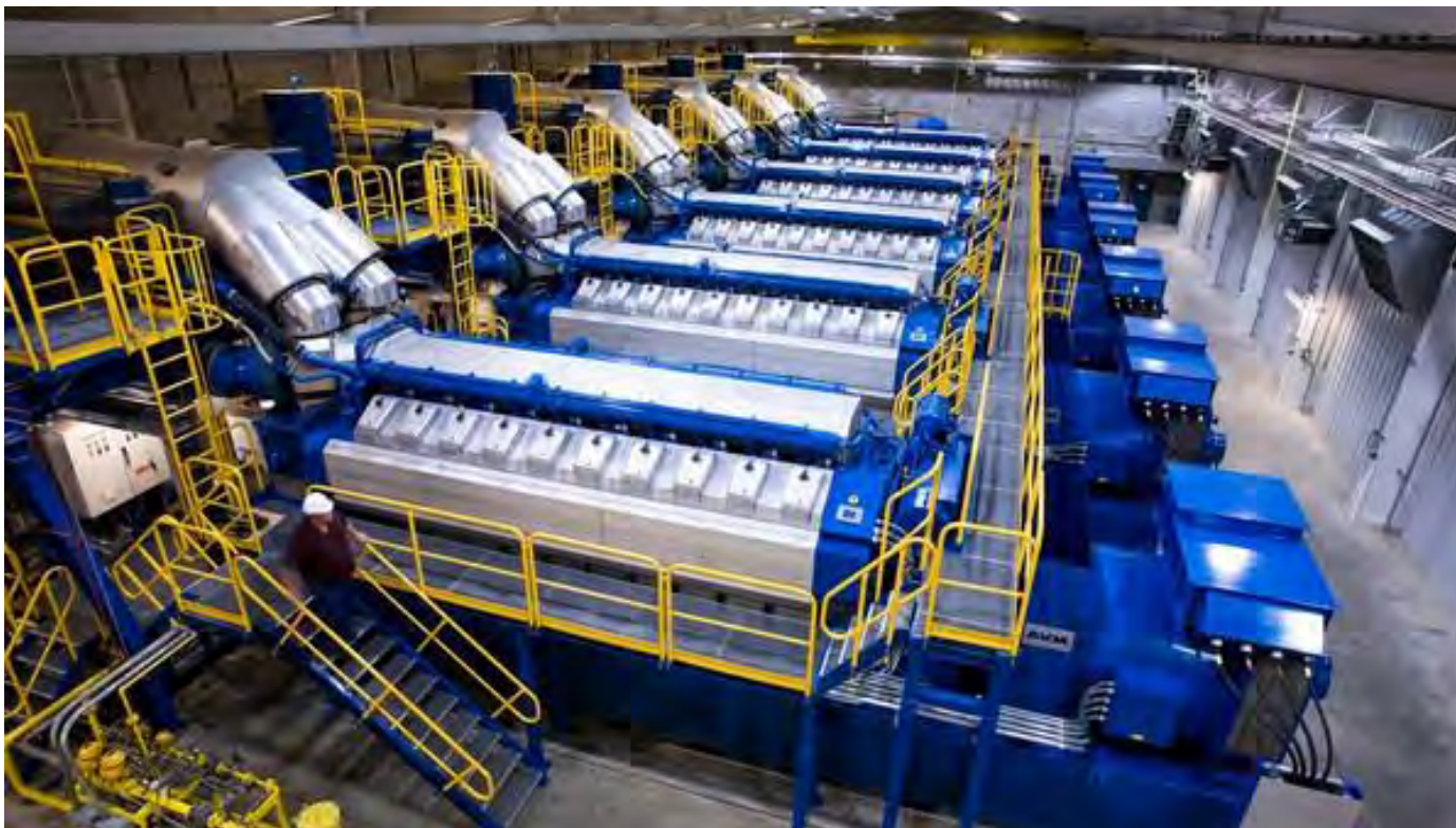
Engine Hall at Goodman Energy Center Kansas
