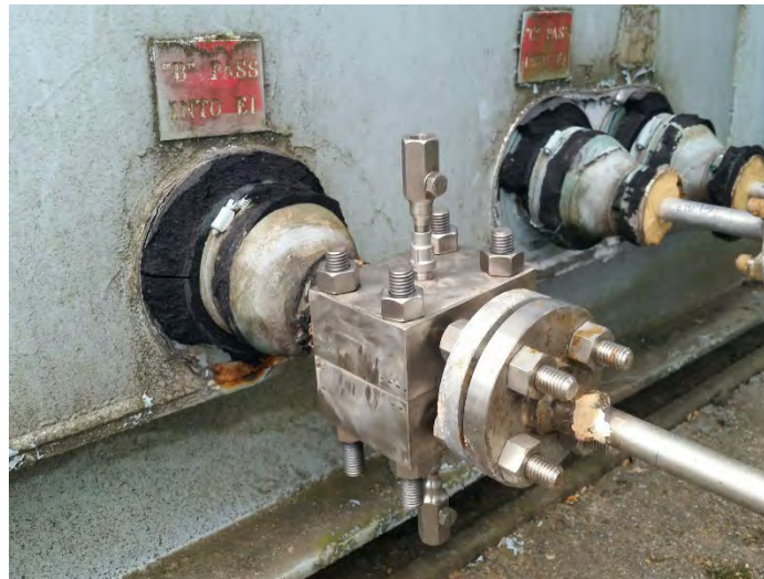
Figure 6.26: Aluminum Pitting Clamp
