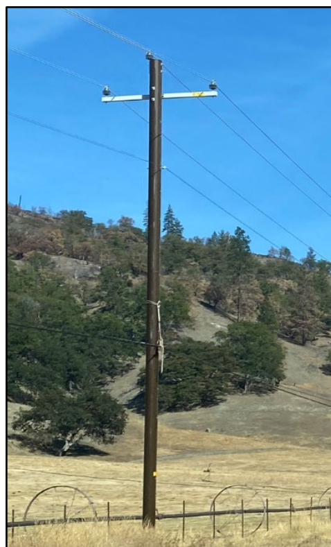
Figure 38: Distribution Fiberglass Poles
