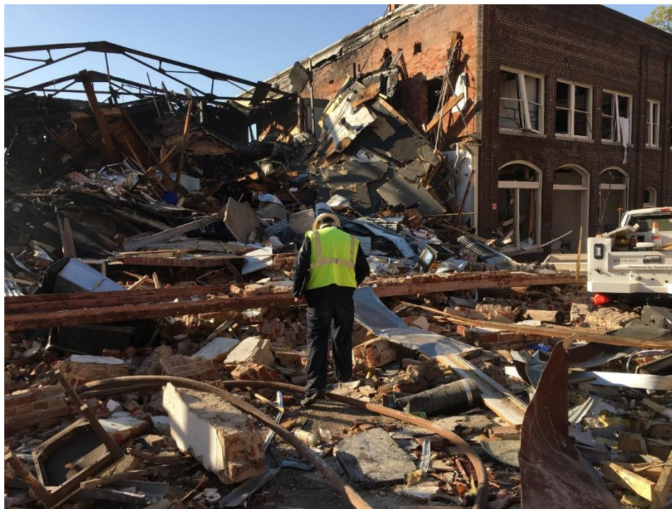
Figure 4: Durham, NC Gas Explosion
