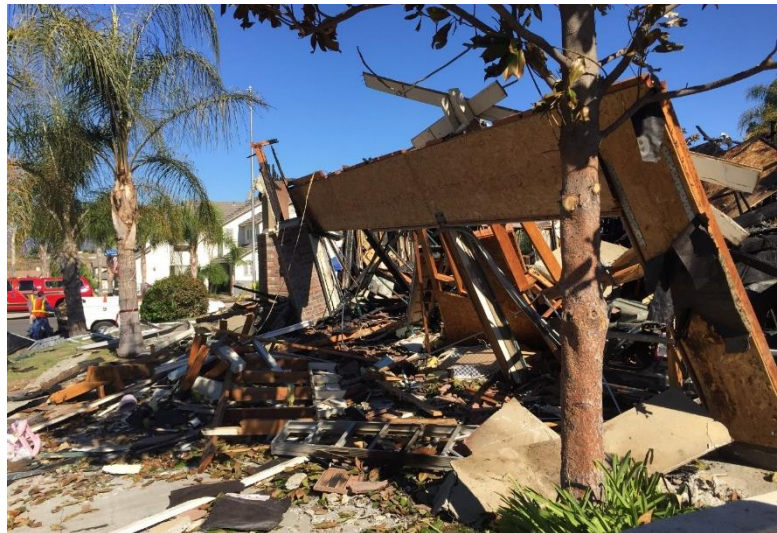
Figure 3: Murrieta, CA Gas Explosion
