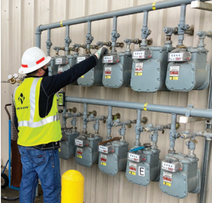
NW Natural technicians testing blended hydrogen gas at NW Natural's Sherwood facility.
