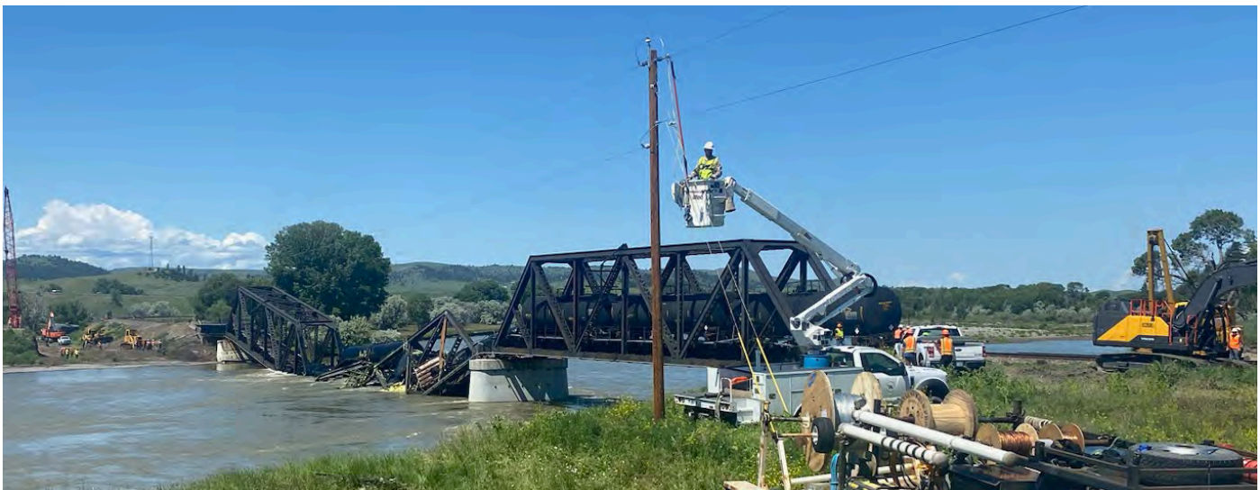
► Rocky Mountain Contractors, an MDU Construction Services Group subsidiary, provided emergency service to repair a long-haul fiber line after a bridge collapsed into the Yellowstone River in Montana.
