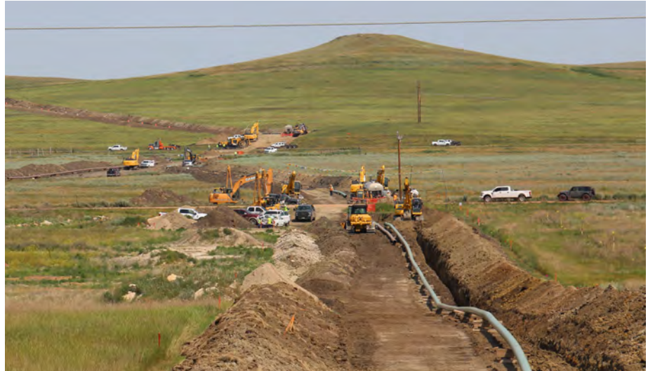
► WBI Energy's Grasslands South Expansion Project was placed into service in November 2023, adding 94 million cubic feet per day of natural gas transportation capacity.
