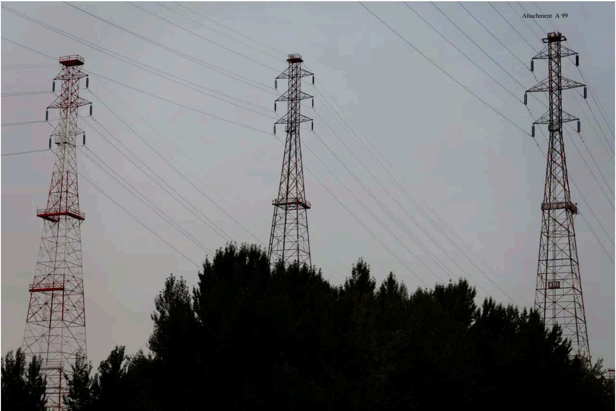
Three high voltage transmission towers, located just south of Sauvie Island, span the Willamette River in Portland, Oregon. LC- The Oregonian
