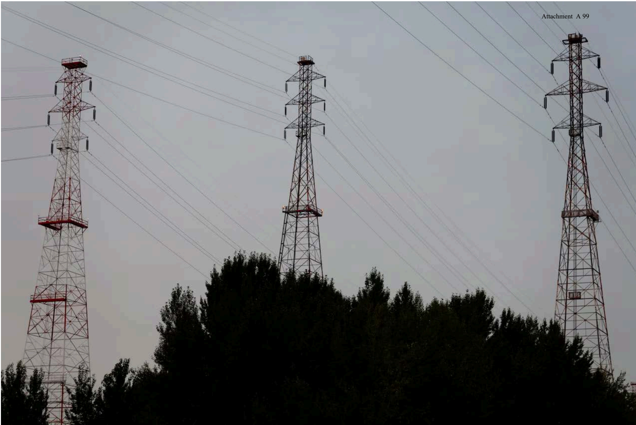
Three high voltage transmission towers, located just south of Sauvie Island, span the Willamette River in Portland, Oregon. LC- The Oregonian
