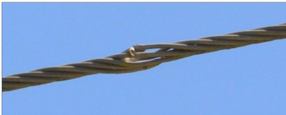
Figure 29. Damaged Conductor Identified by EFD System
