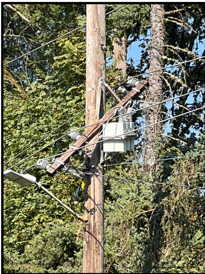
Figure 16: Damage to Distribution Pole, September 2022 PSPS Event
