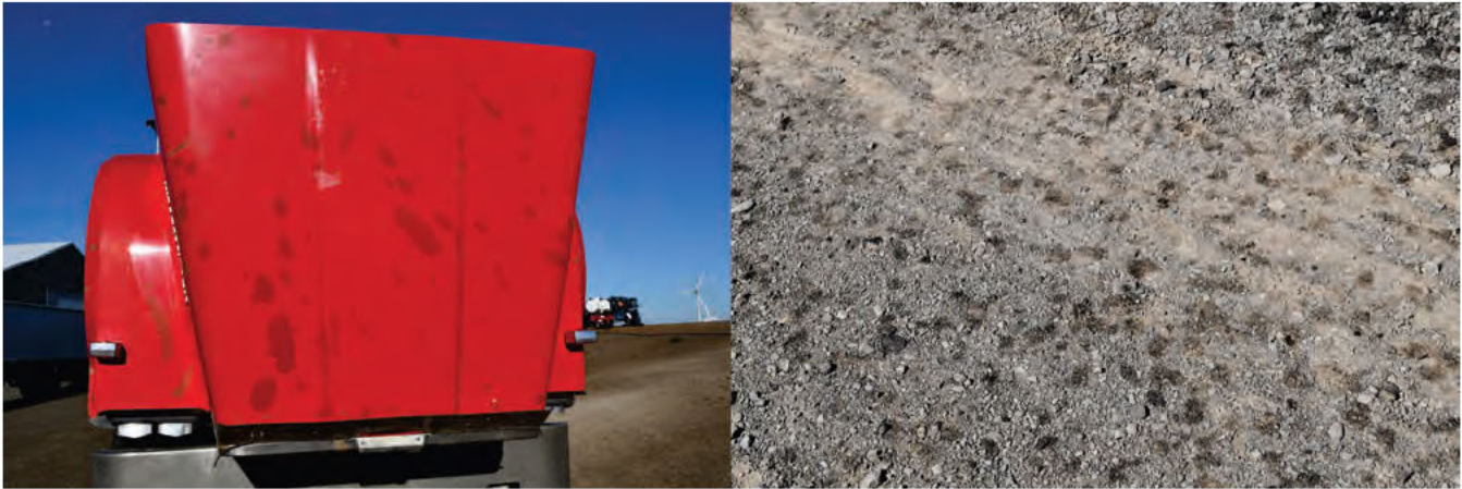
Kevin McCullough parked his truck near one of Biglow Canyon's Vestas wind turbines for about 30 minutes during wheat harvest in early August. When he returned, he said it was spattered in oil leaking from the top of the turbine. At right, oil spots on the ground nearby the same turbine. Landowners worry that regular leaks of oil and lubricants from Vestas turbines, which PGE says is a fixable problem if it chooses to make the investment, could be contaminating their cropland. (Courtesy Kathryn McCullough)
