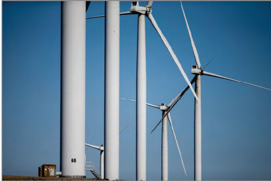
Residents who own land under PGE's Biglow Canyon wind farm worry that regular leaks of oil and lubricants from turbines pose fire and environmental hazards.
