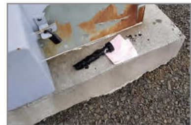
A broken blade bolt found under a wind turbine at Biglow Canyon wind farm by a worker delivering fertilizer in late January. A day or two later, the turbine threw an eight-ton blade into a nearby field. (Courtesy Kevin Massie)
