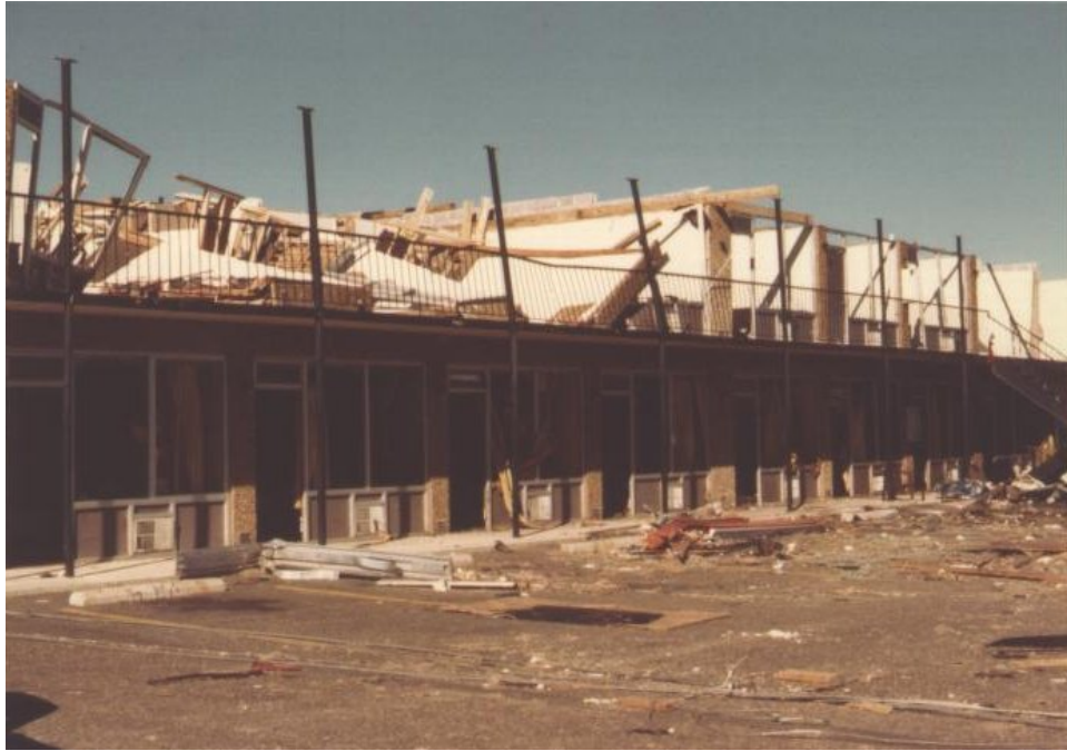
MAM: DOD 5: Collapse of top story walls
