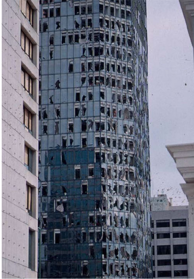
HRB: DOD 8: Broken glass in curtain wall; significant damage to building interior
