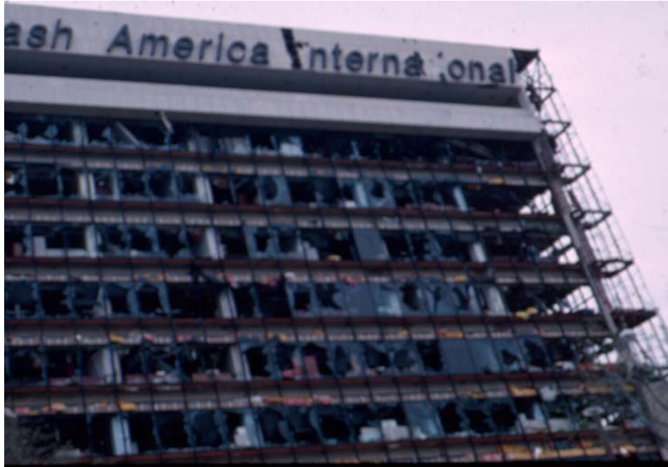
MRB: DOD 9: Significant damage to curtain walls and some interior walls
