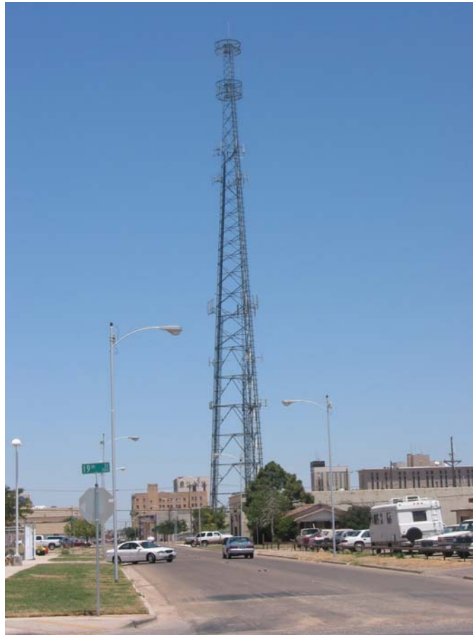
FST: Free-standing Truss Tower
