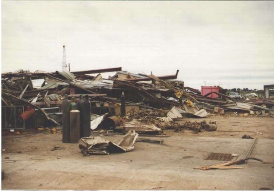
MBS: DOD 8: Total destruction of building
