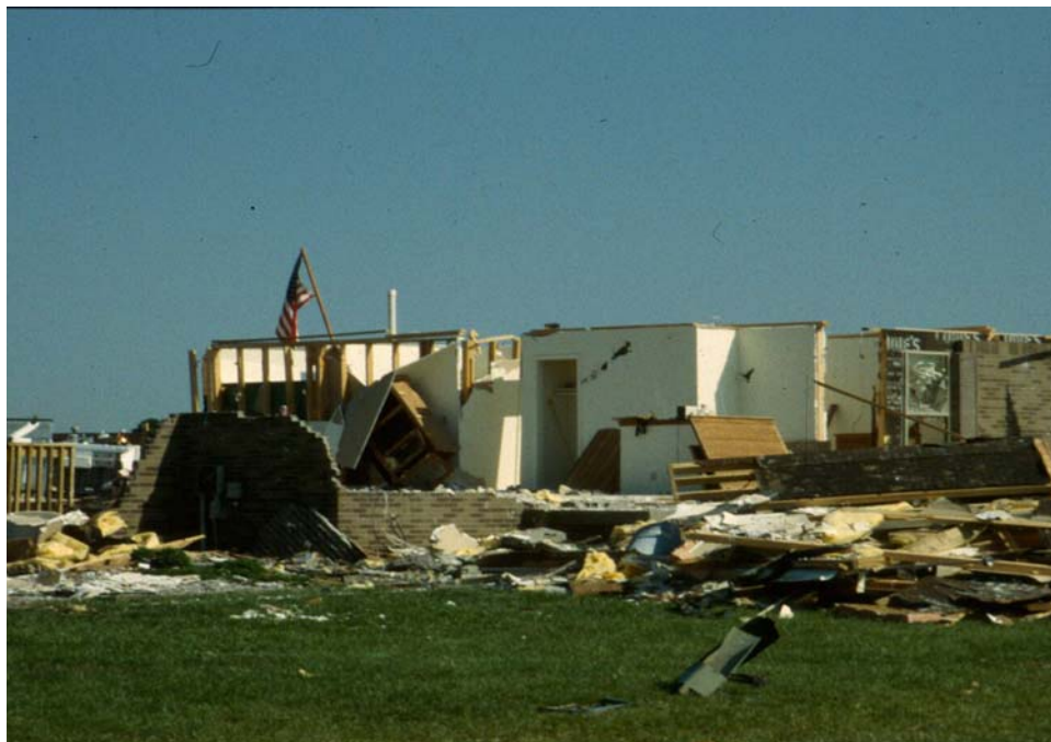
FR12: DOD 7: Top floor (First floor in this case) exterior walls collapsed
