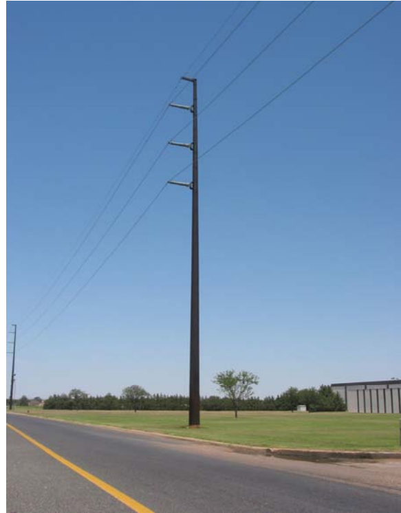
ETL: Single Steel Pole
