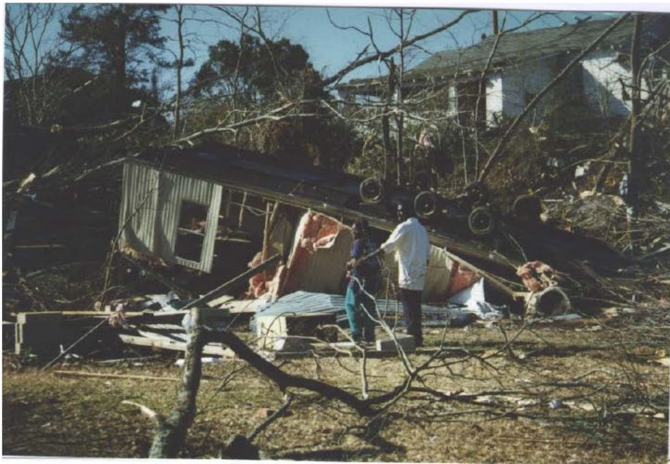
MHSW: DOD 9: Complete destruction of unit; debris blown away
