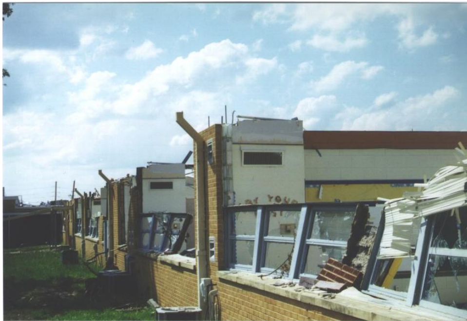
ES: DOD 8: Uplift of entire roof structure and collapse of non-bearing walls
