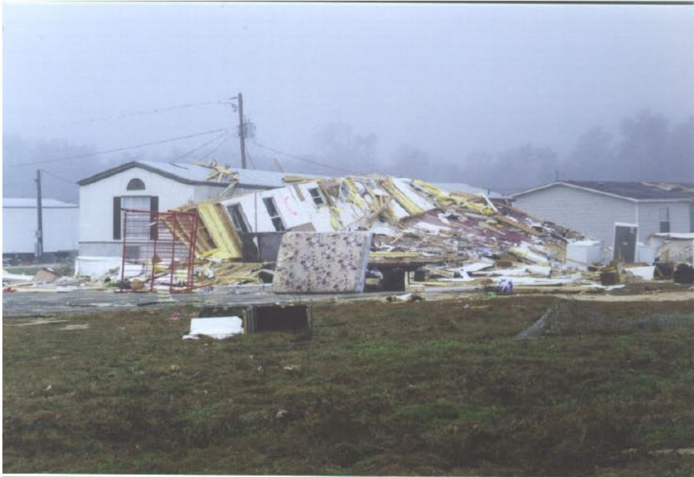
MHSW: DOD 6: Destruction of roof and walls leaving floor and undercarriage in place
