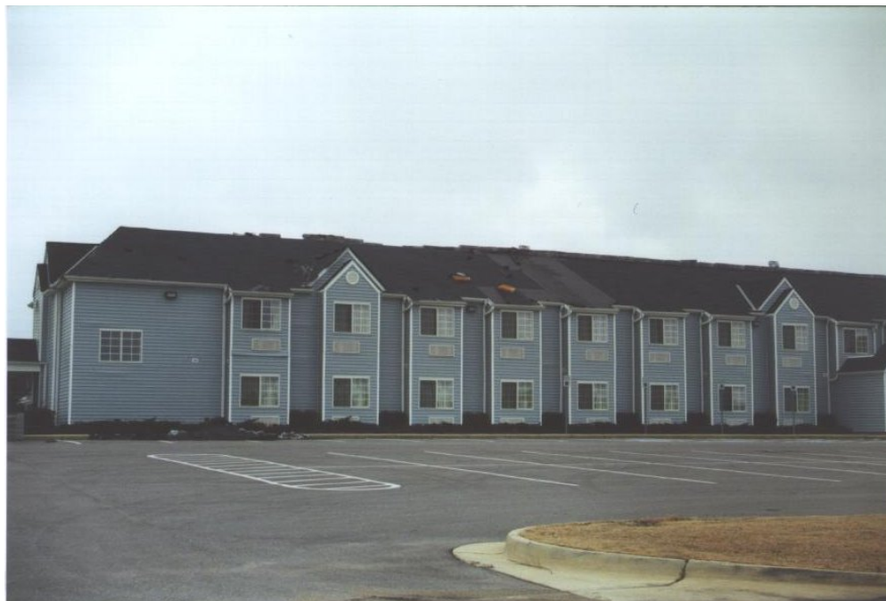
ACT: DOD 2: Loss of roof covering (<20%)
