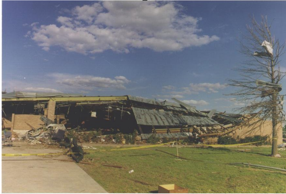
ES: DOD 9: Collapse of load-bearing walls
