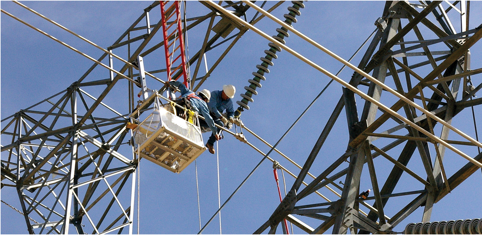
Repair of insulator on 345-kV tower Bonanza- Mona line. Photo courtesy of Deseret Power Electric Cooperative
