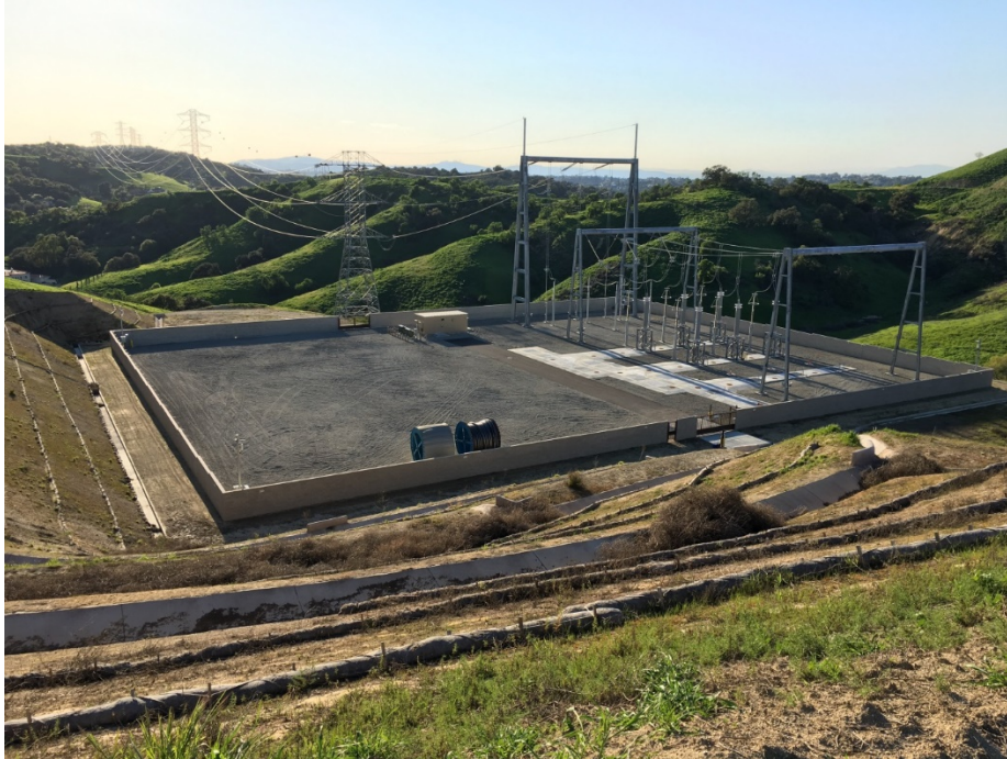
Figure 10: Chino Hill's 500 kV Transition Station
