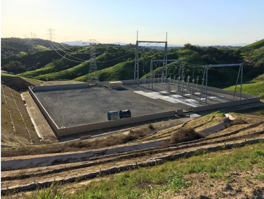
Figure 1: Chino Hills 500 kV Transition Station
