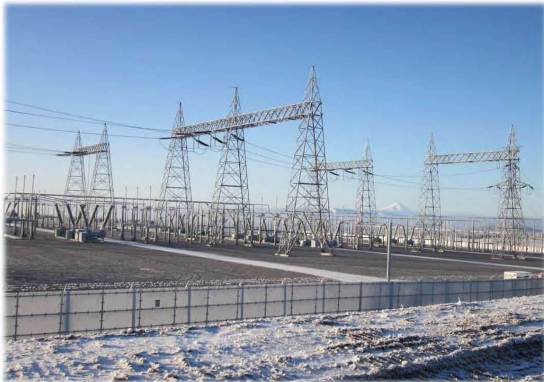
Figure 2-12. Typical 500-kV Substation
