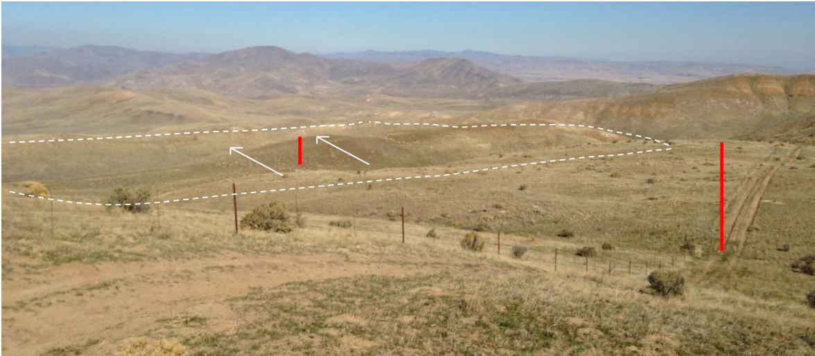
Photo 3: Looking north into the landslide complex; approximate locations of towers 205/2 and 205/3 shown for reference.
