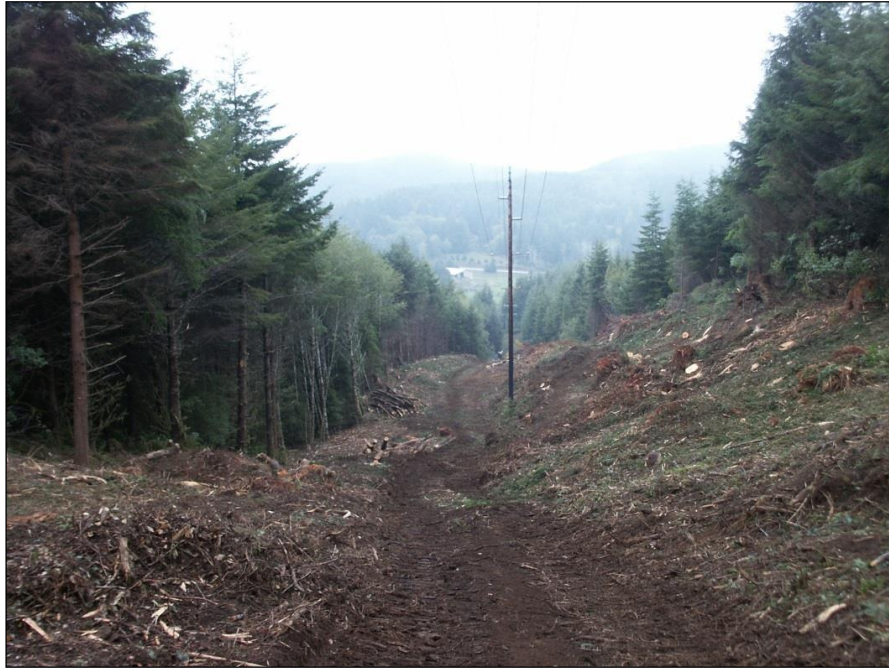
Figure 6.2. Line 4 in California following work (note the trees mid-span where the line is more than 100-feet off the ground).
