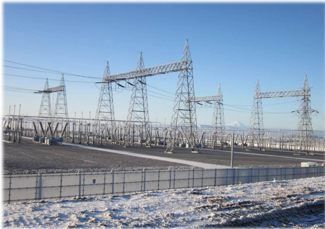
Figure 2-12. Typical 500-kV Substation
