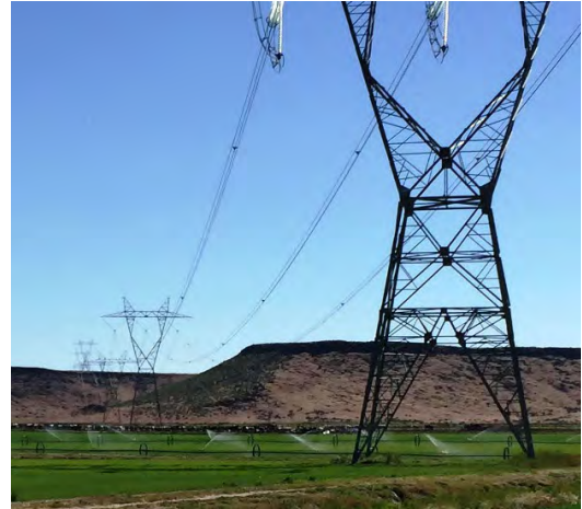
500-kilovolt (kV) transmission line near Melba, Idaho
