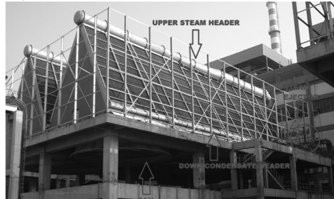
Fig. 4 Air Cooled condenser components (Ultratech Power plant)
