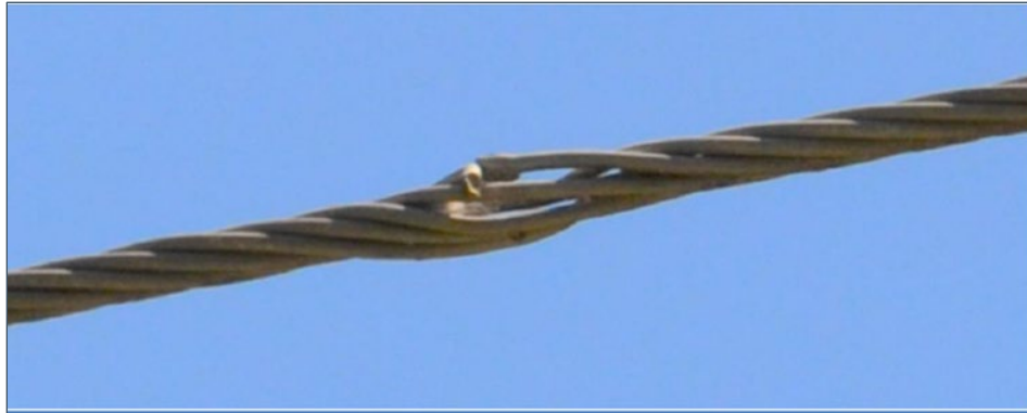
Figure 29. Damaged Conductor Identified by EFD System
