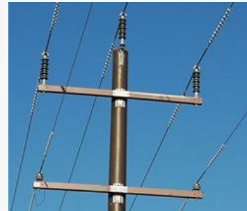
Ductile iron poles & covered wire
