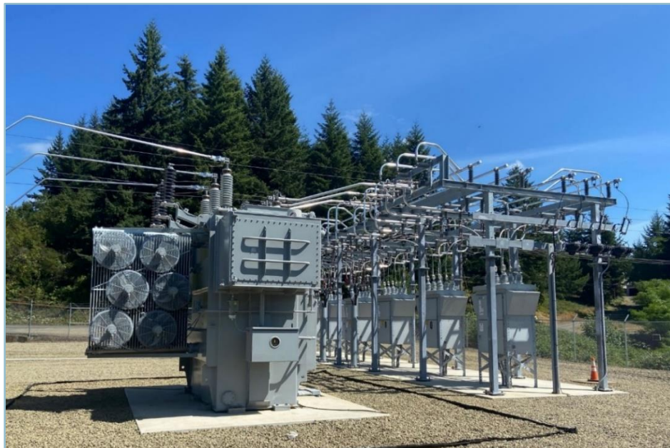
Central Lincoln crews construct and maintain the utility's substations
