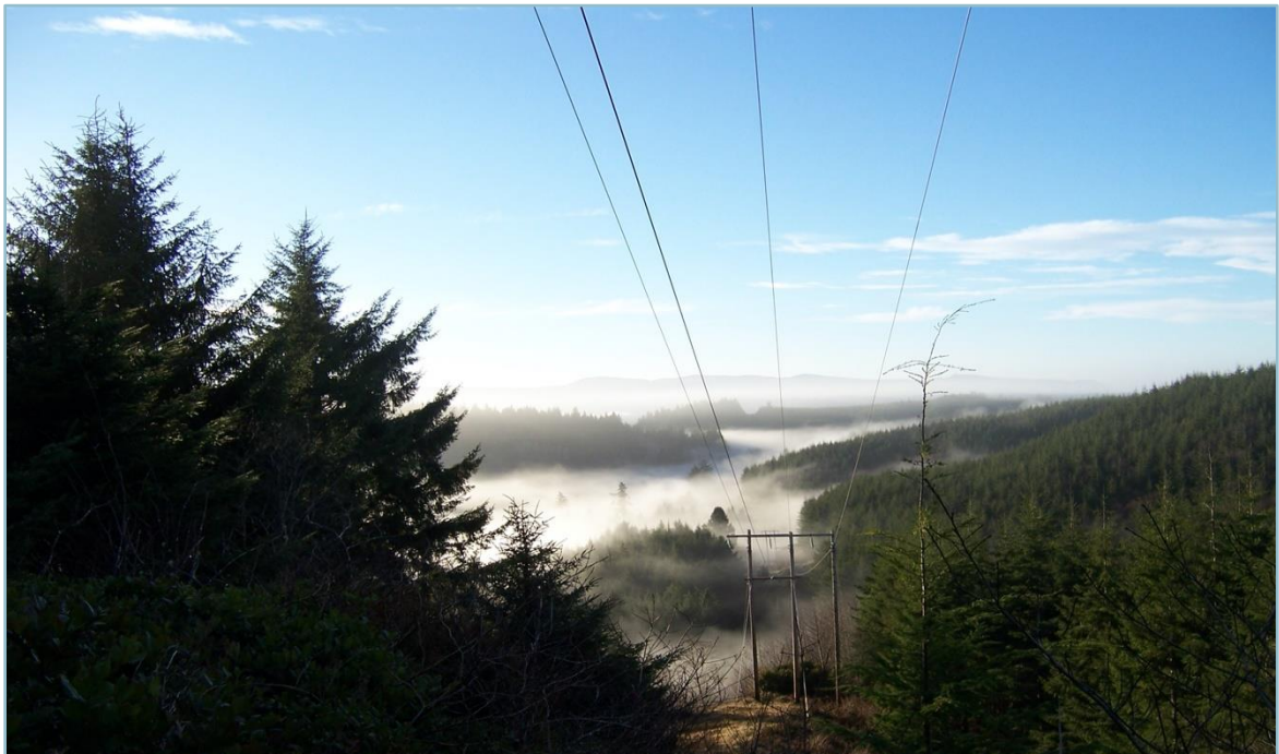
Central Lincoln transmission line
