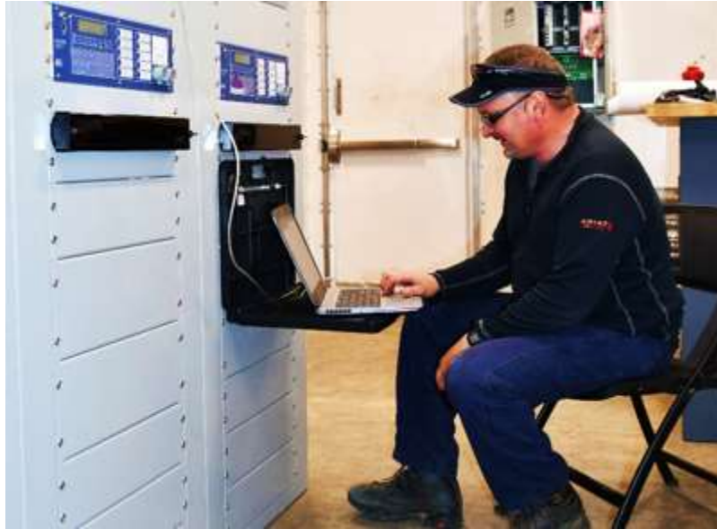
CRPUD serviceman adjusting substation settings
