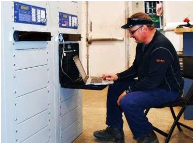
CRPUD serviceman adjusting substation settings
