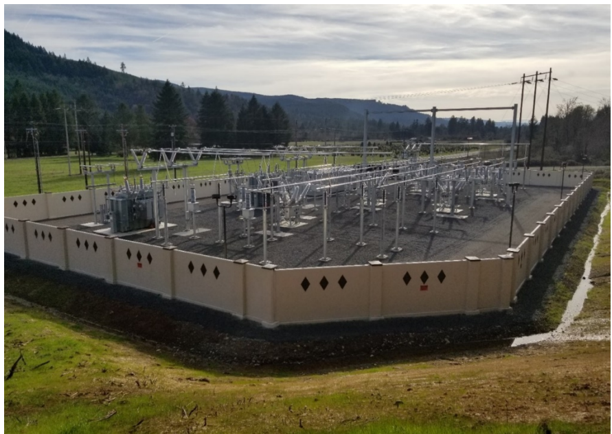
Holden Creek Substation
