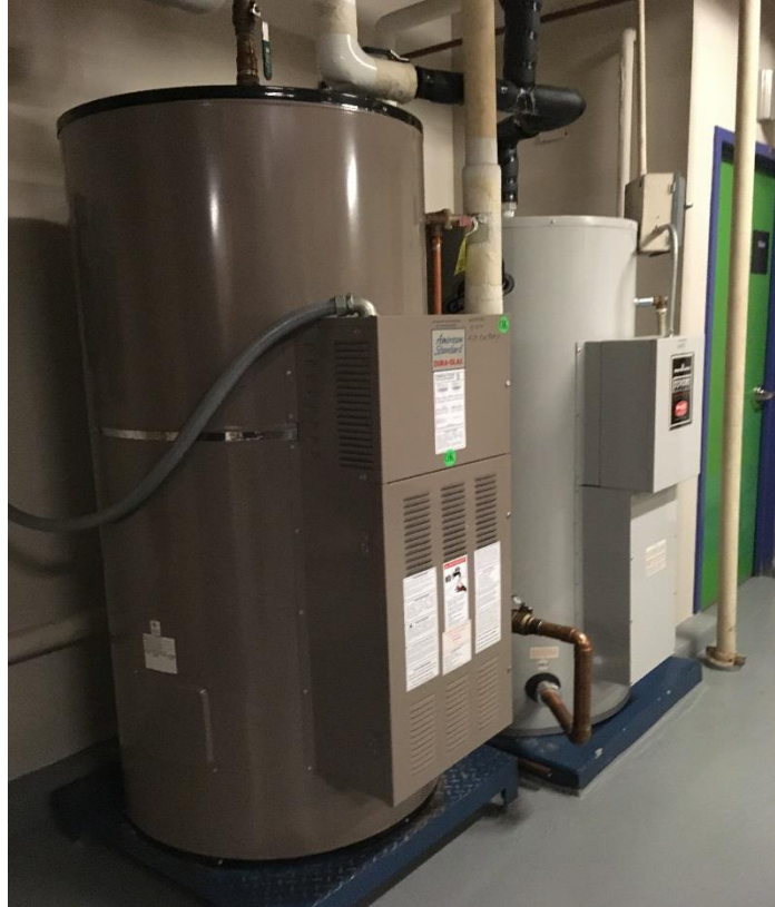
Unbraced Water Heaters at P1 Level
