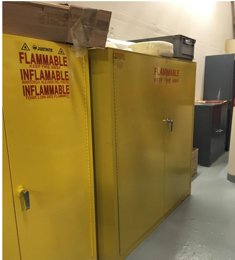
Unbraced Flammable Materials Cabinet at P1 Level
