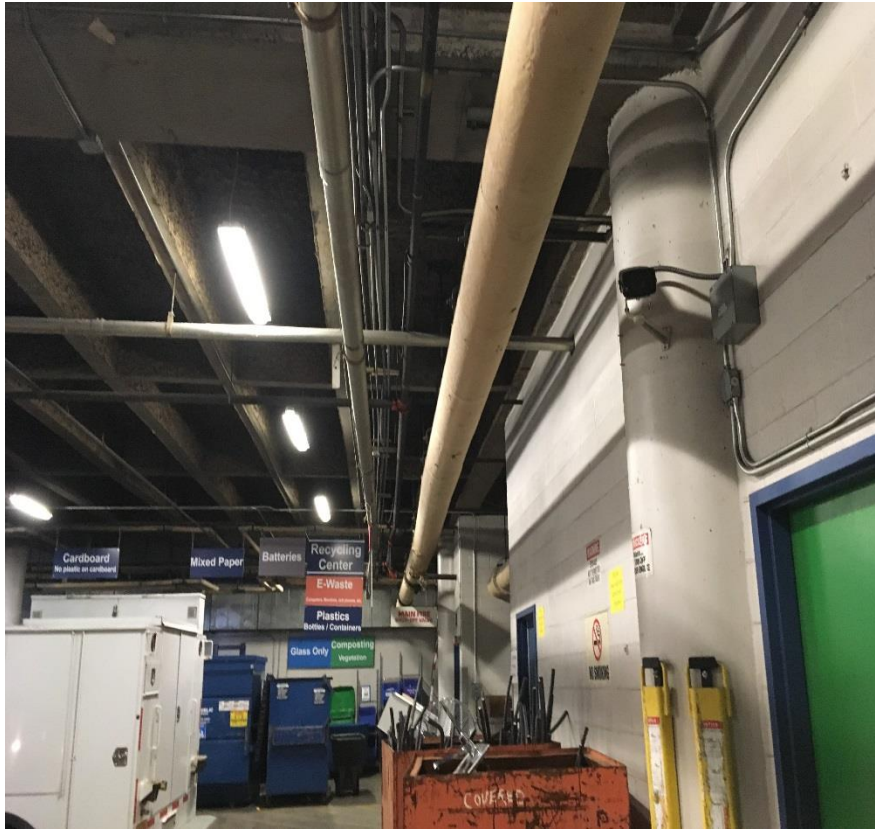
Unbraced Piping Run at P1 Level
