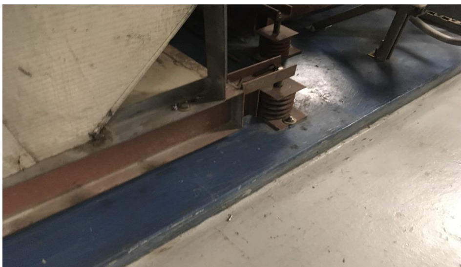
Vibration Isolators Lacking Snubbers
