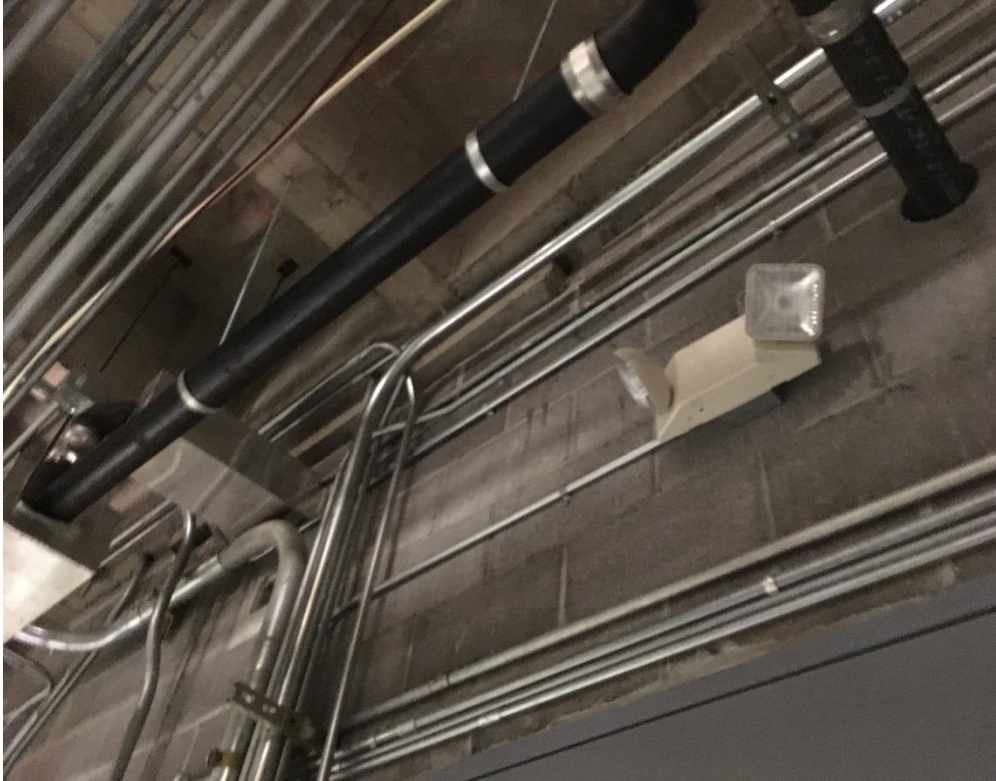
Unbraced CMU Partition Wall at Level P1
