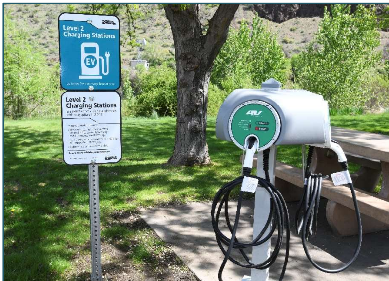
Figure 4 Copperfield Campground Level 2 EV Charging Port
