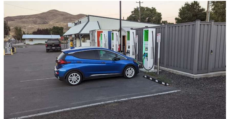
Electrify America Charging Station: Huntington, Oregon
