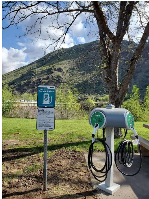
Level 2 EV Charger: Copperfield Campground
