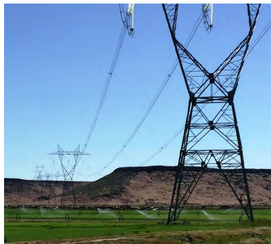
500-kilovolt (kV) transmission line near Melba, Idaho
