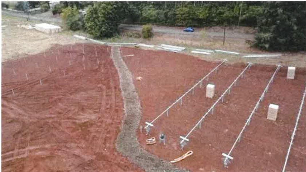
Auburn Solar as of September 26, 2023
