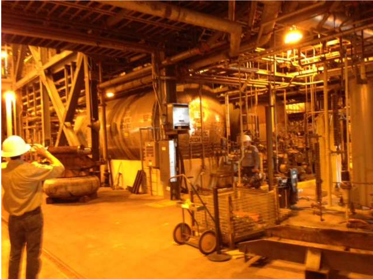
Sodium Hydroxide tank (left near ground), Sulfuric Acid tank (center), Soda Ash tank on the right
