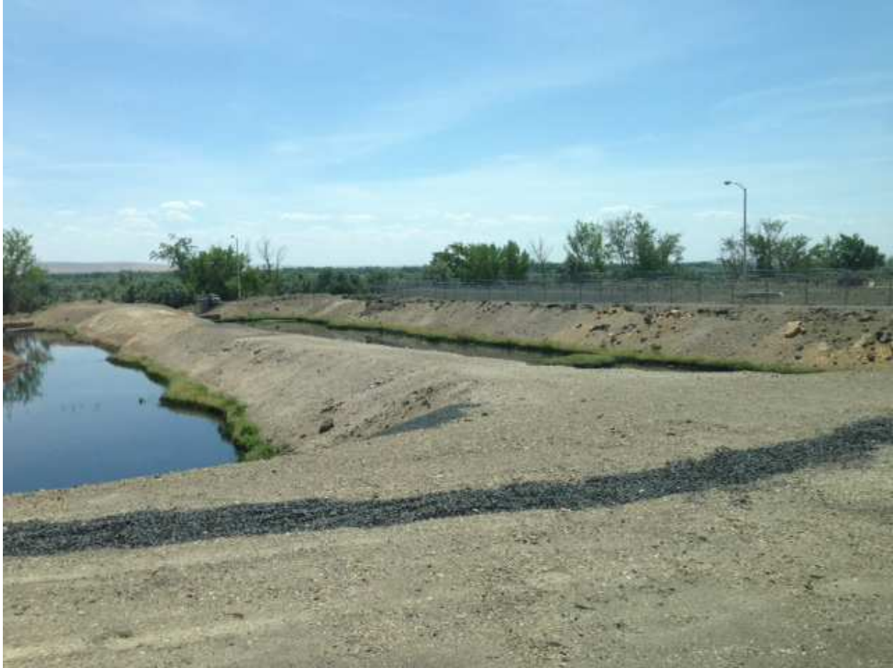
Settling Ponds, west & east, gravel ribbon is a French drain to keep surface runoff from eroding the pond walls
