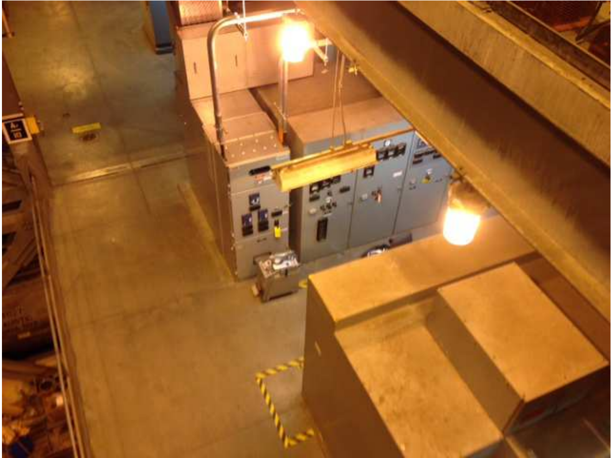
Looking down through the crane bay at switch gear on the second floor
