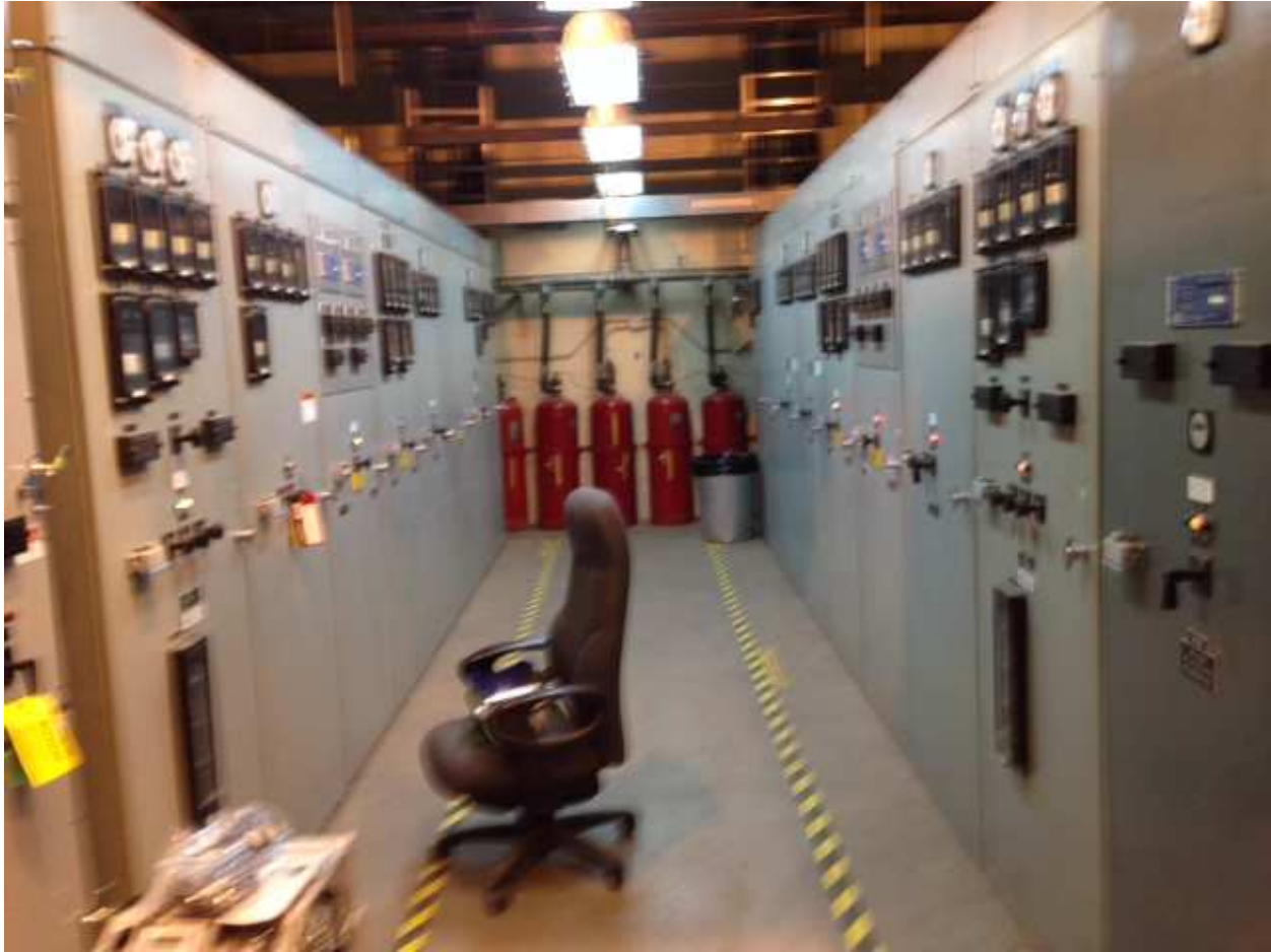
2d floor, more breakers, HALON bottles at the end wall
