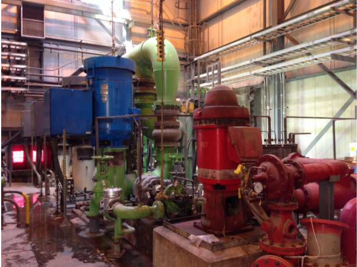
Electric fire water pump (in red)
