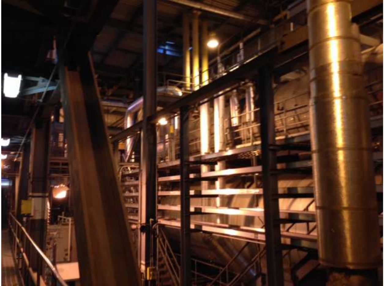
DA heater on top, DA storage tank below
