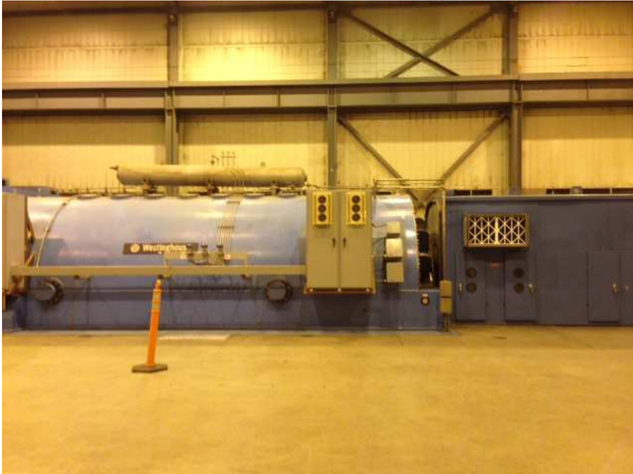
Generator and exciter enclosures
