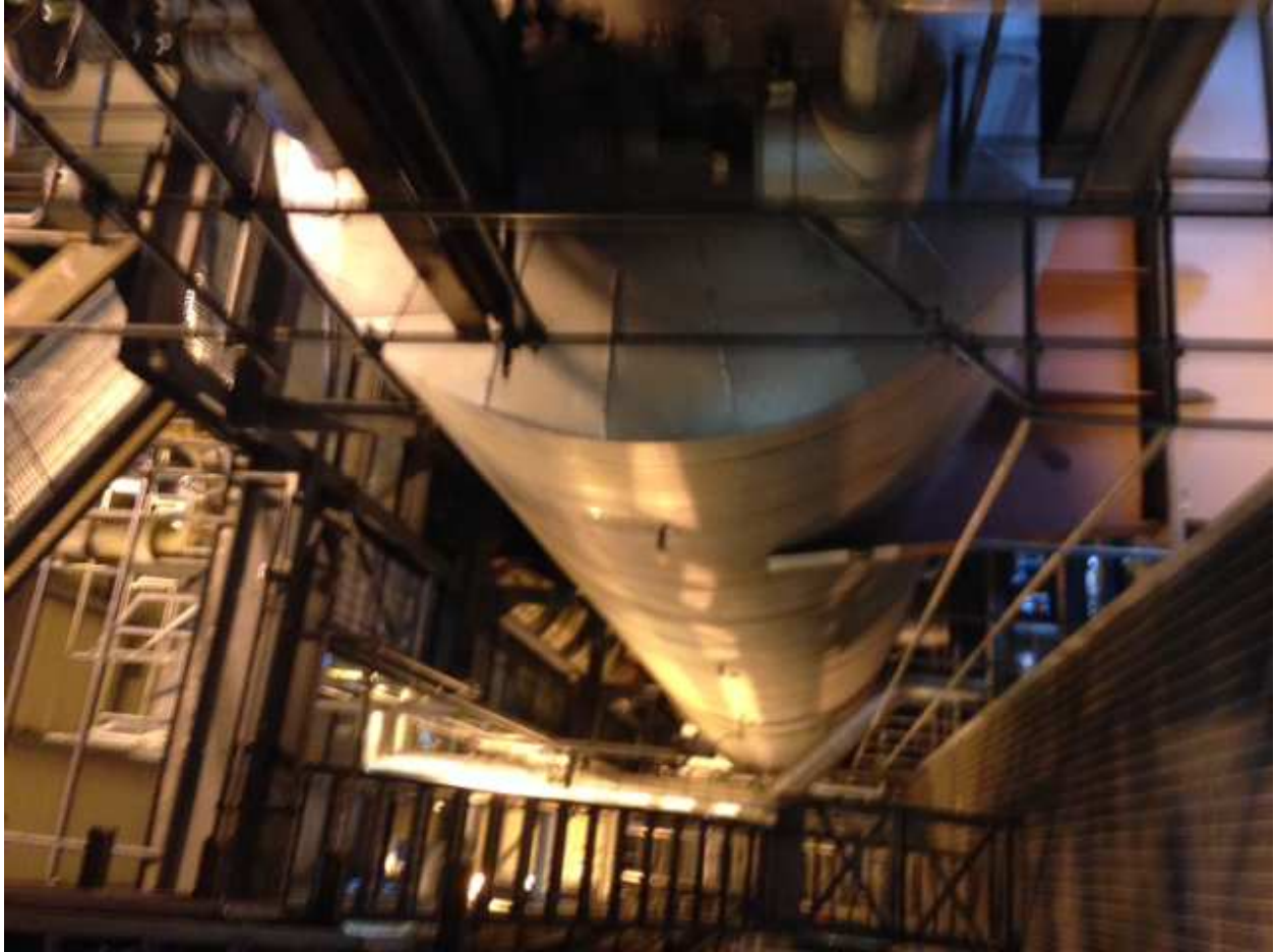
Deaerator (DA) storage tank (9 th floor)
