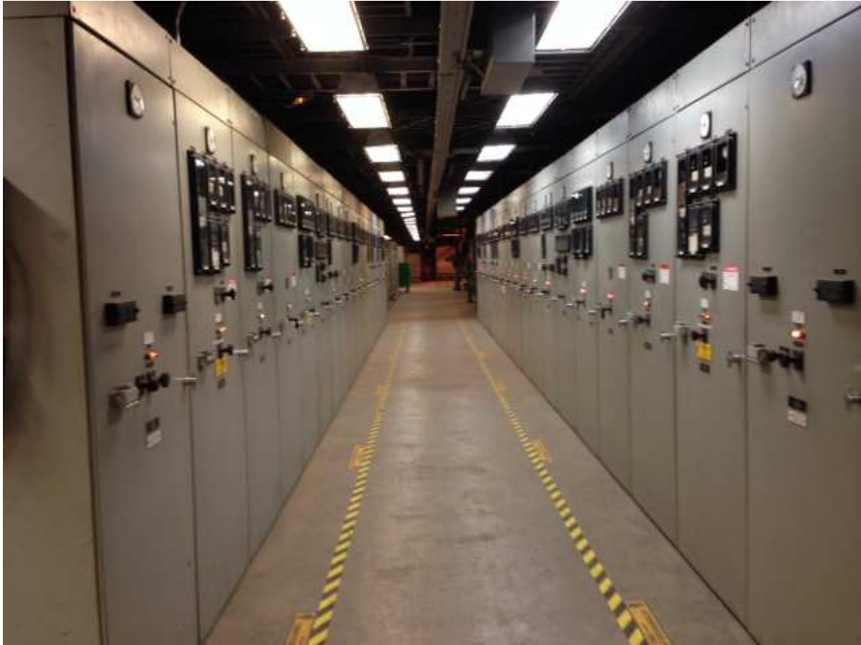
7.2 Kv breakers for big motors everywhere
