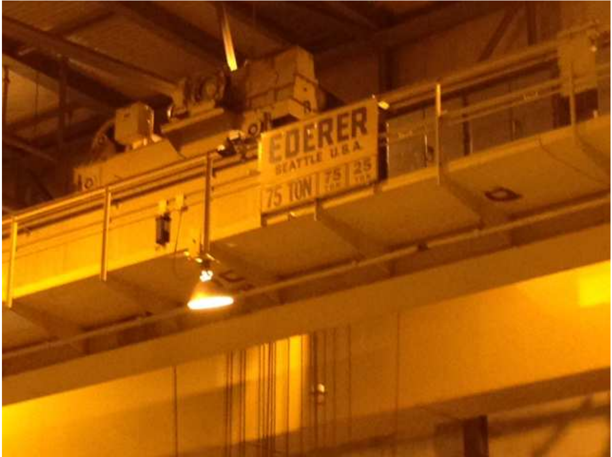
Turbine deck overhead trolley crane
