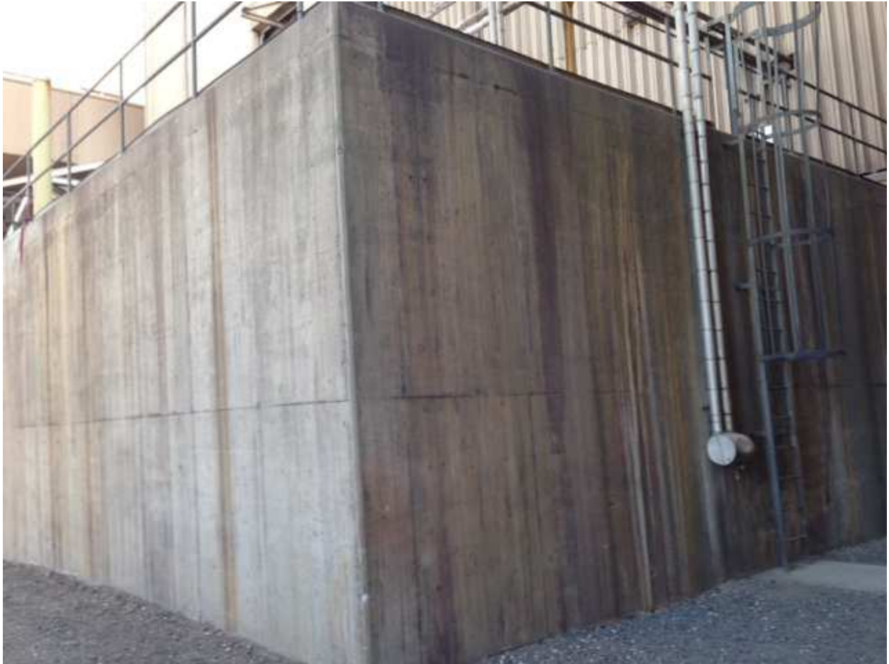
Neutralization sump (there is as much underground as there is above ground)
