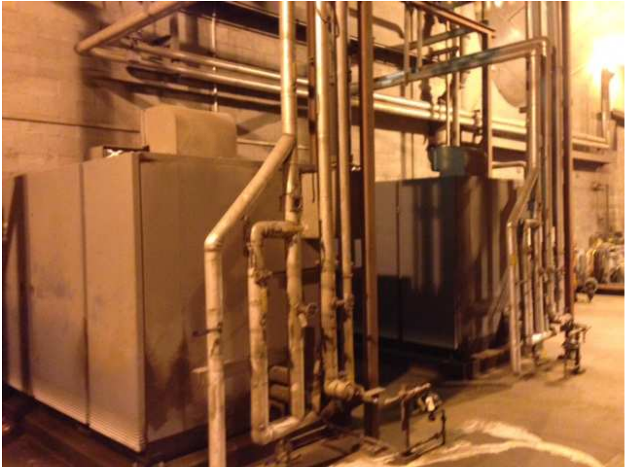
COPCO soot blowing air compressors (currently a backup system)
