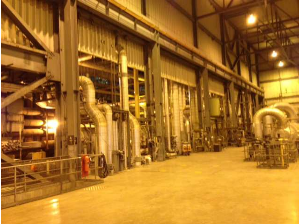
Turbine deck. FWH #3 on the right, pipe race on the left
