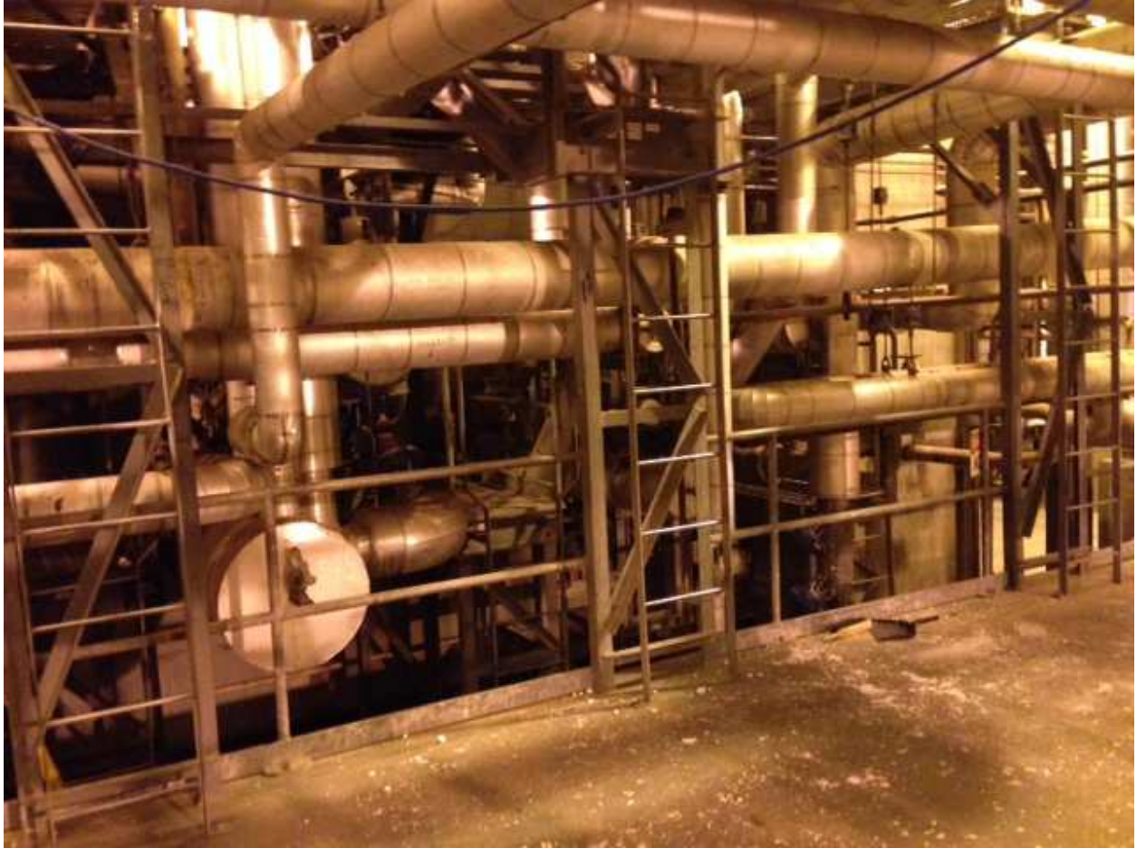
Condensate pit (south view)
