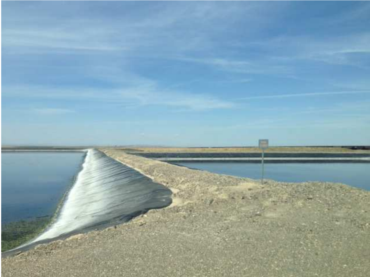
Dike between 10 Ac evaporation pond and 2 Ac evaporation pond. There is a French drain type leak detection drain below the base of the dike
