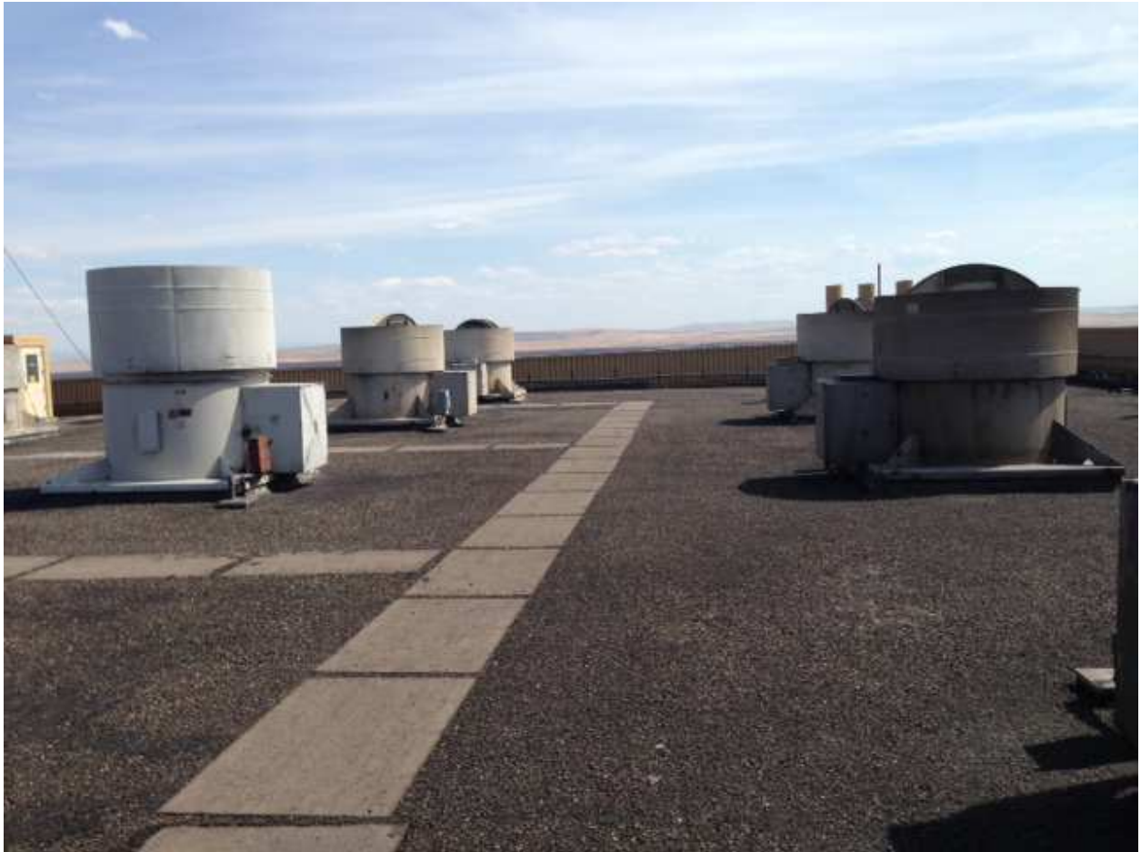
Power block roof with ventilation fans
