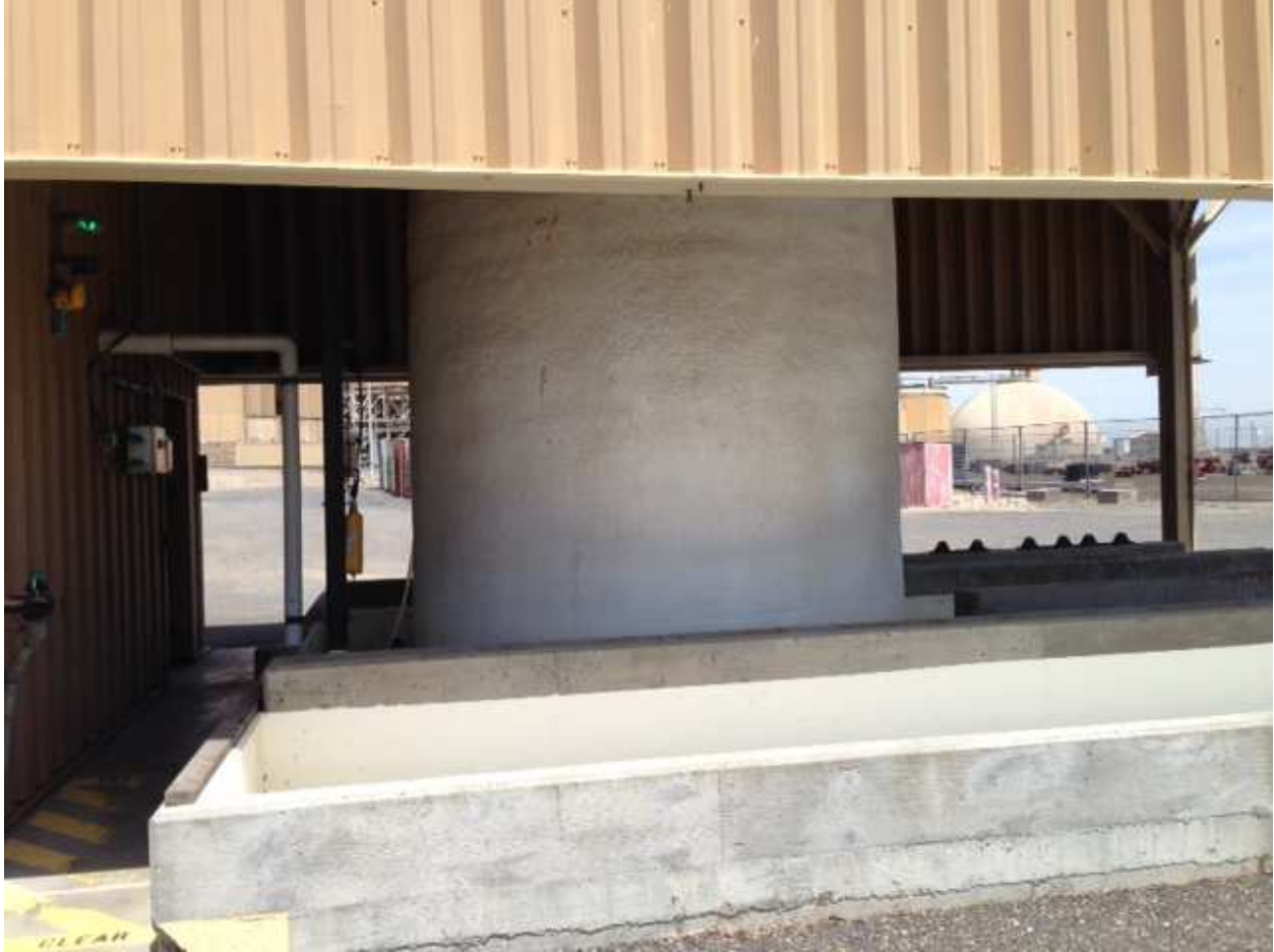
NaOCl tank for chlorination for Circulation and Service water, 6000 gal, polyethylene
