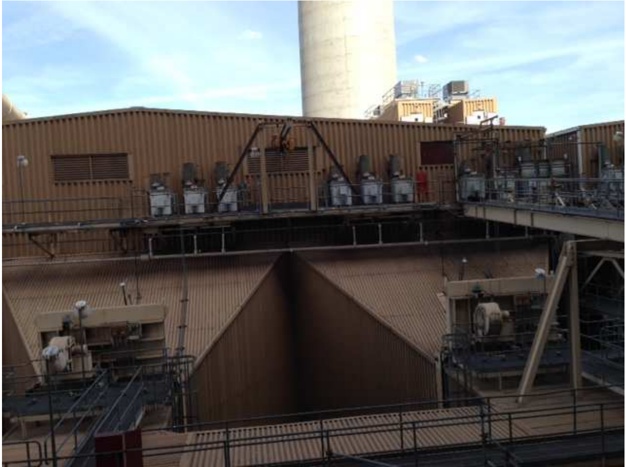
ESP inlet nozzles, B1 & B2, T/R sets on the catwalk
