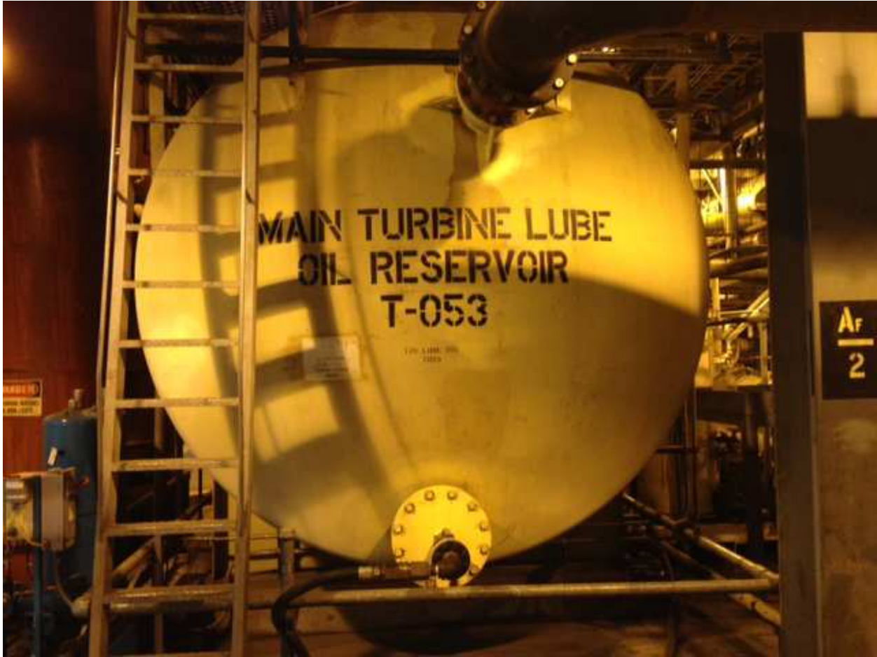
Main Turbine Lube Oil reservoir
