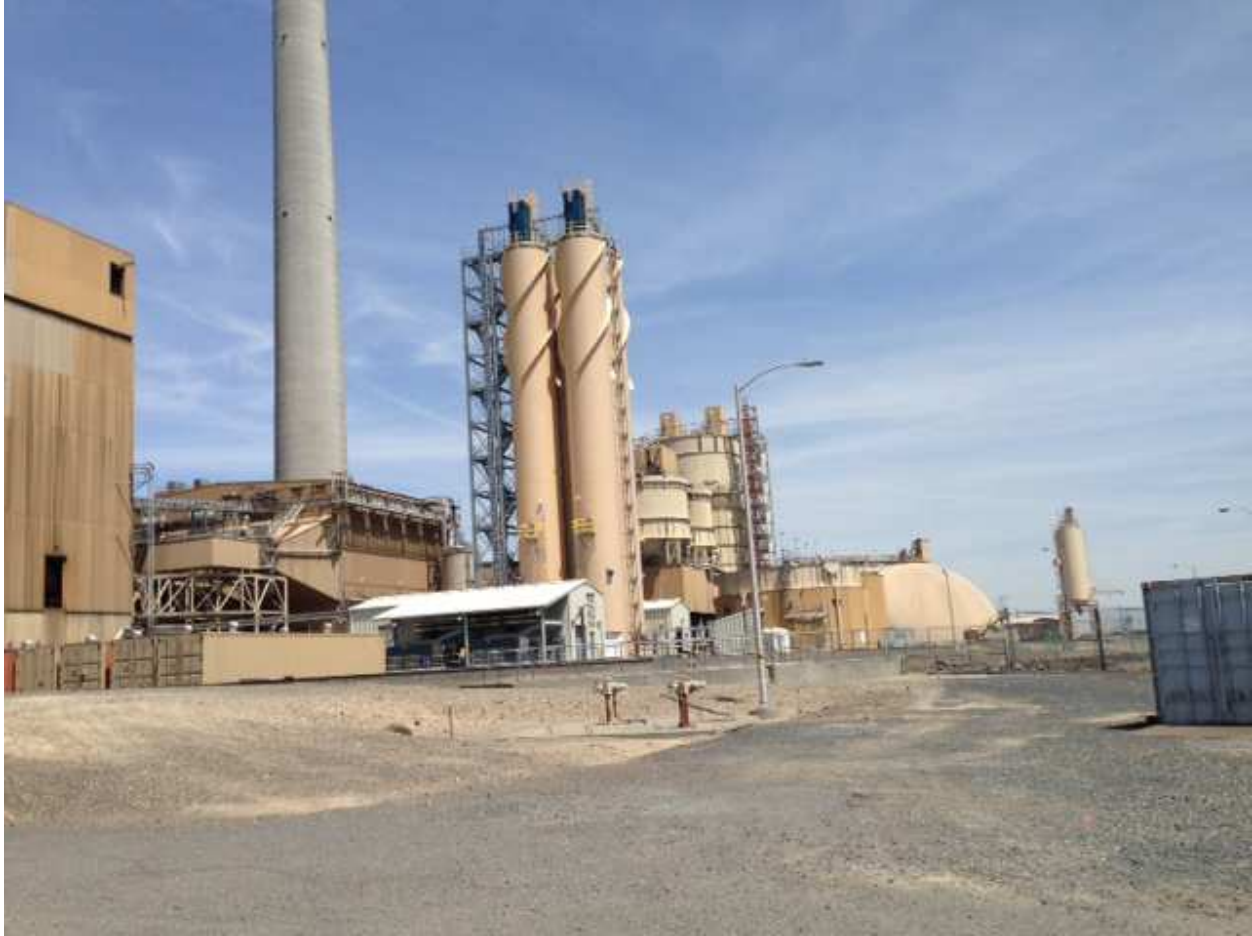
Trona silos and DSI facility with reservoir make up valve pit in the foreground
