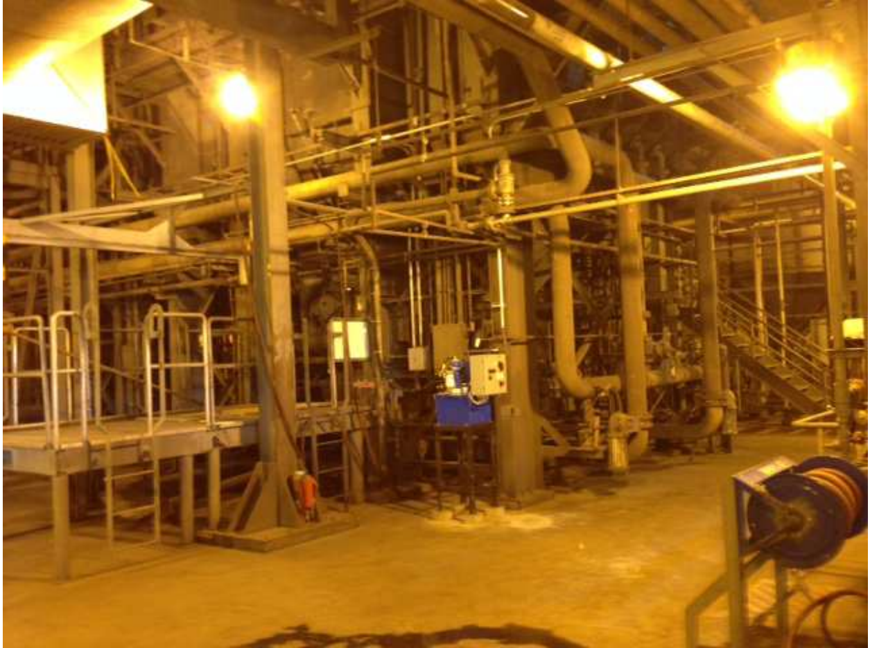
West Bottom Ash Hopper area
