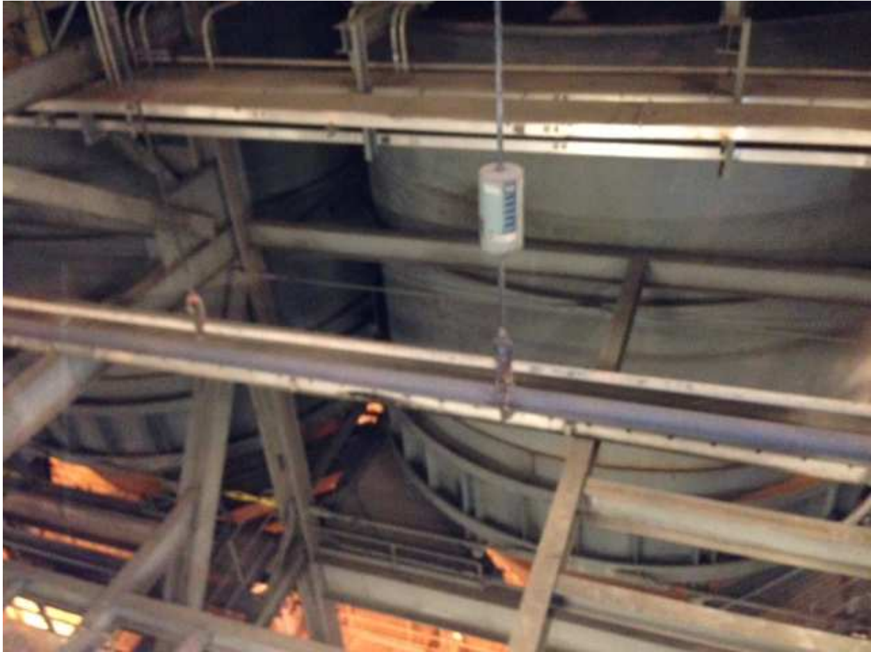
Spring hanger in front of a coal silo
