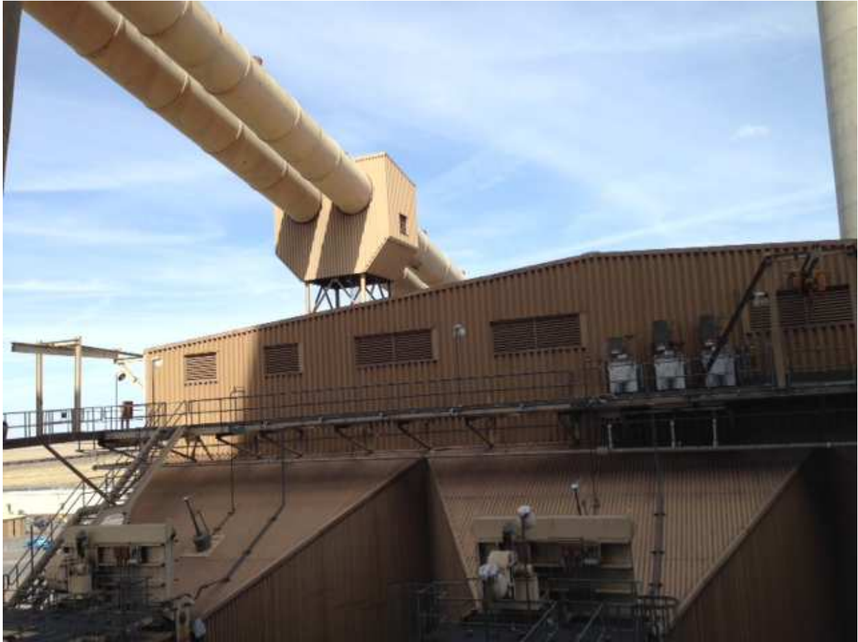
ESP inlet nozzles, B2 & B3
