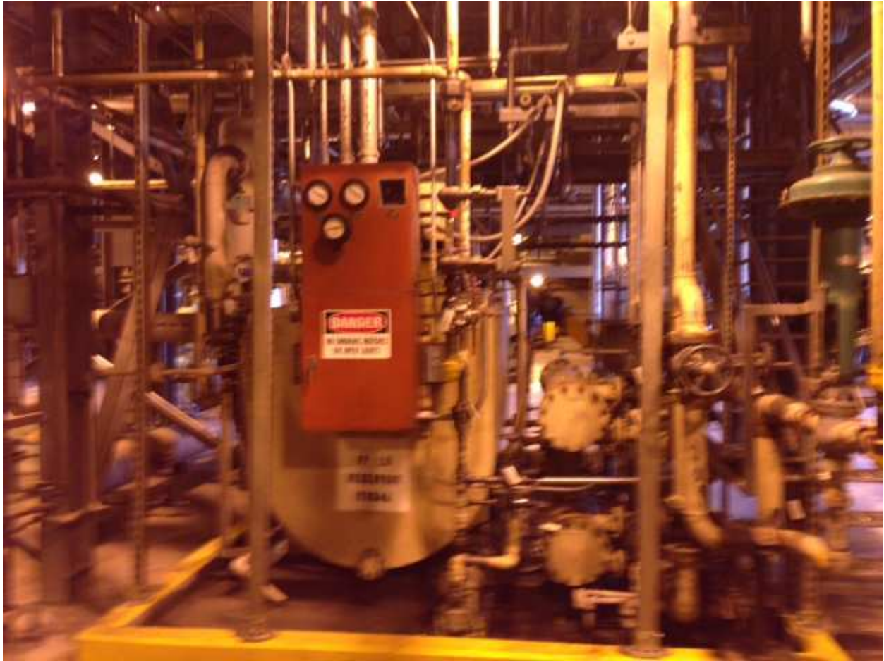
FPT lube oil reservoir
