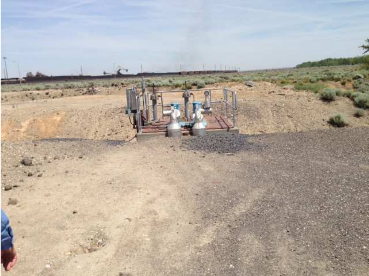
Settling ponds sump pumps A & B
