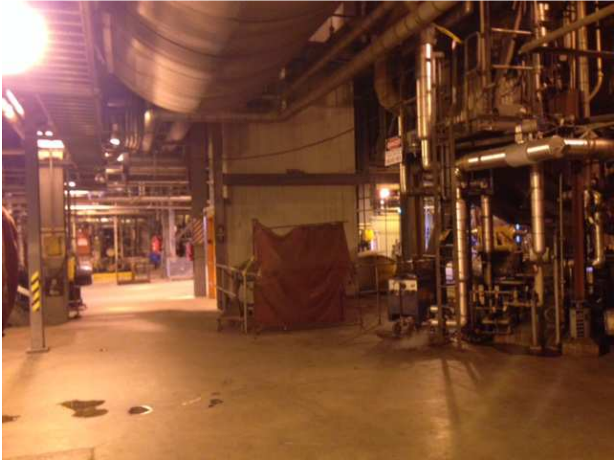
PA duct overhead in north pulverizer row
