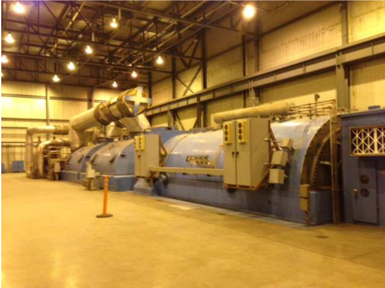
Turbine deck. l <-> r HP/IP turbine, LP1 turbine, LP2 turbine, generator, exciter
