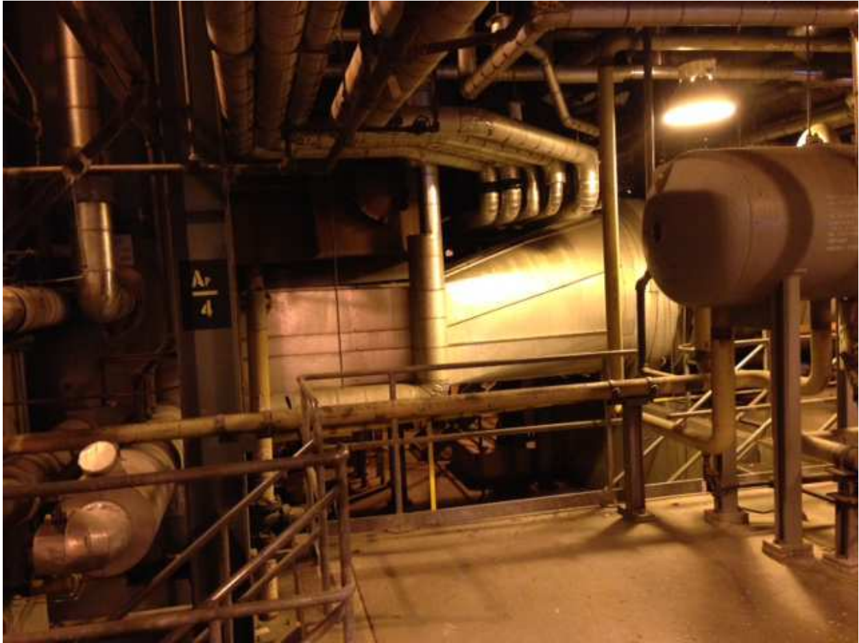
South Feed Pump Turbine
