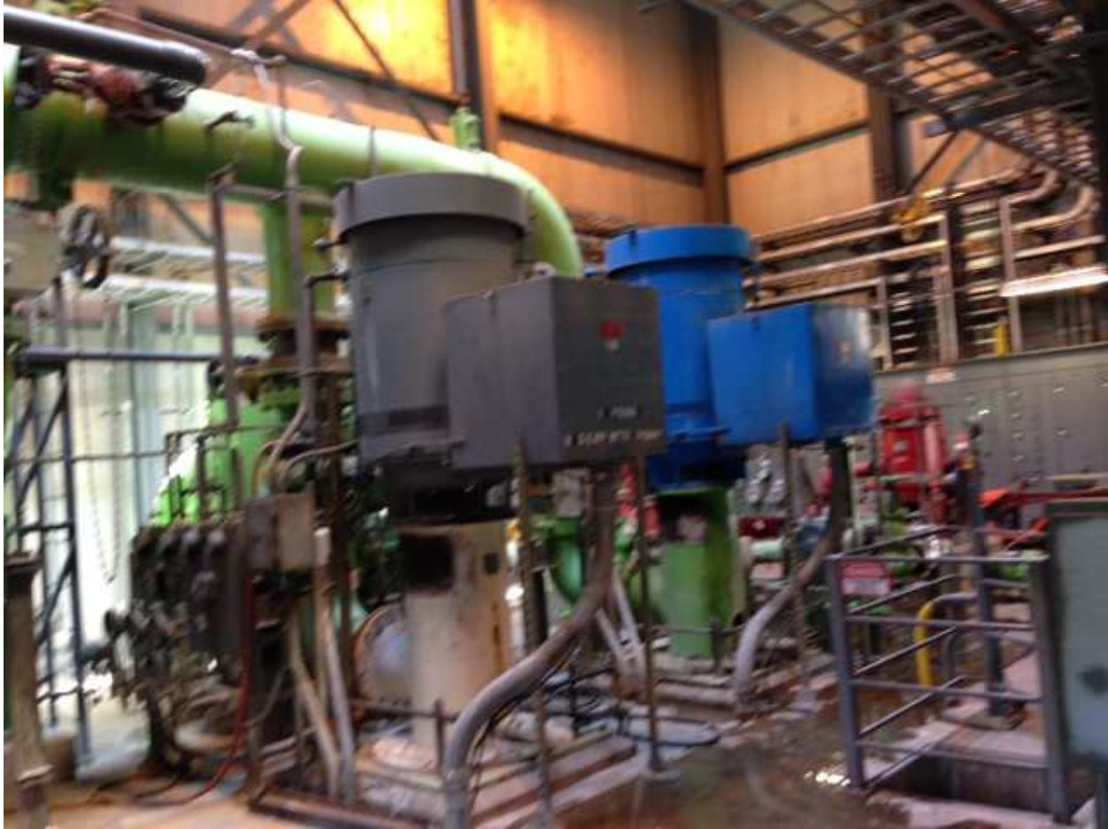
Service Water pump/motor (B&C pumps) inside the Intake Structure Building
