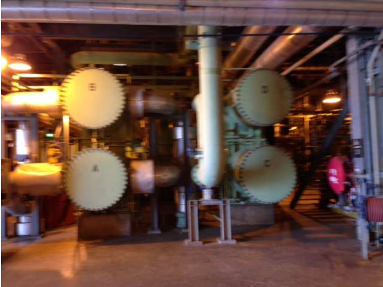
Aux Cooling Water Heat Exchangers (A,B,C,&D)
