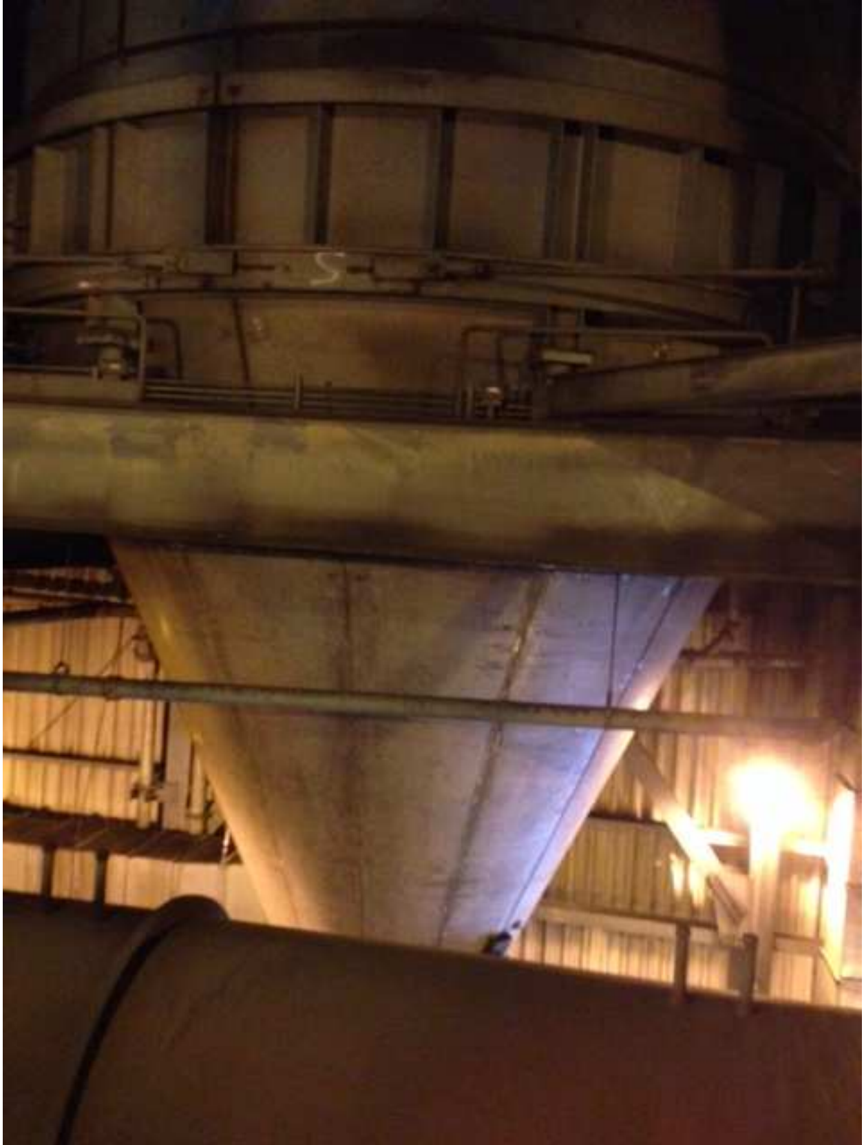
Coal silo cone, sloped part is stainless
