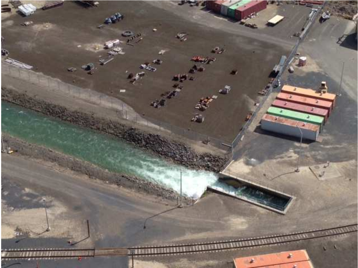
Circulation water discharge seal structure, lay down yard and storage CONEX boxes
