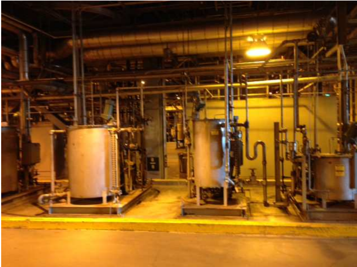
Boiler chemical injection skid. Includes 1/2 of the Ammonium Hydroxide tank, Hydrazine tank, Phosphate tank, Aux Boiler tank
