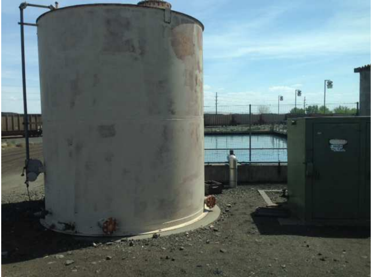
surfactant tank (abandoned in place)
