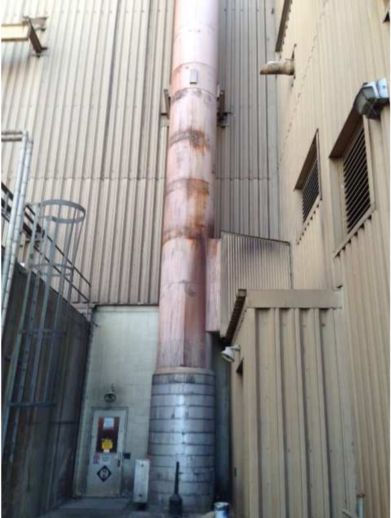
Aux Boiler stack
