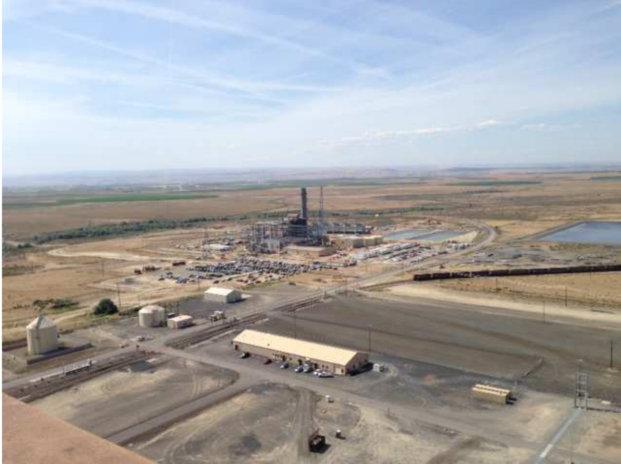
Oil storage tank (peaked roof), Fire water storage tank (dome roof), sheet metal shop/MPC bldg. (long), and gas plant construction
