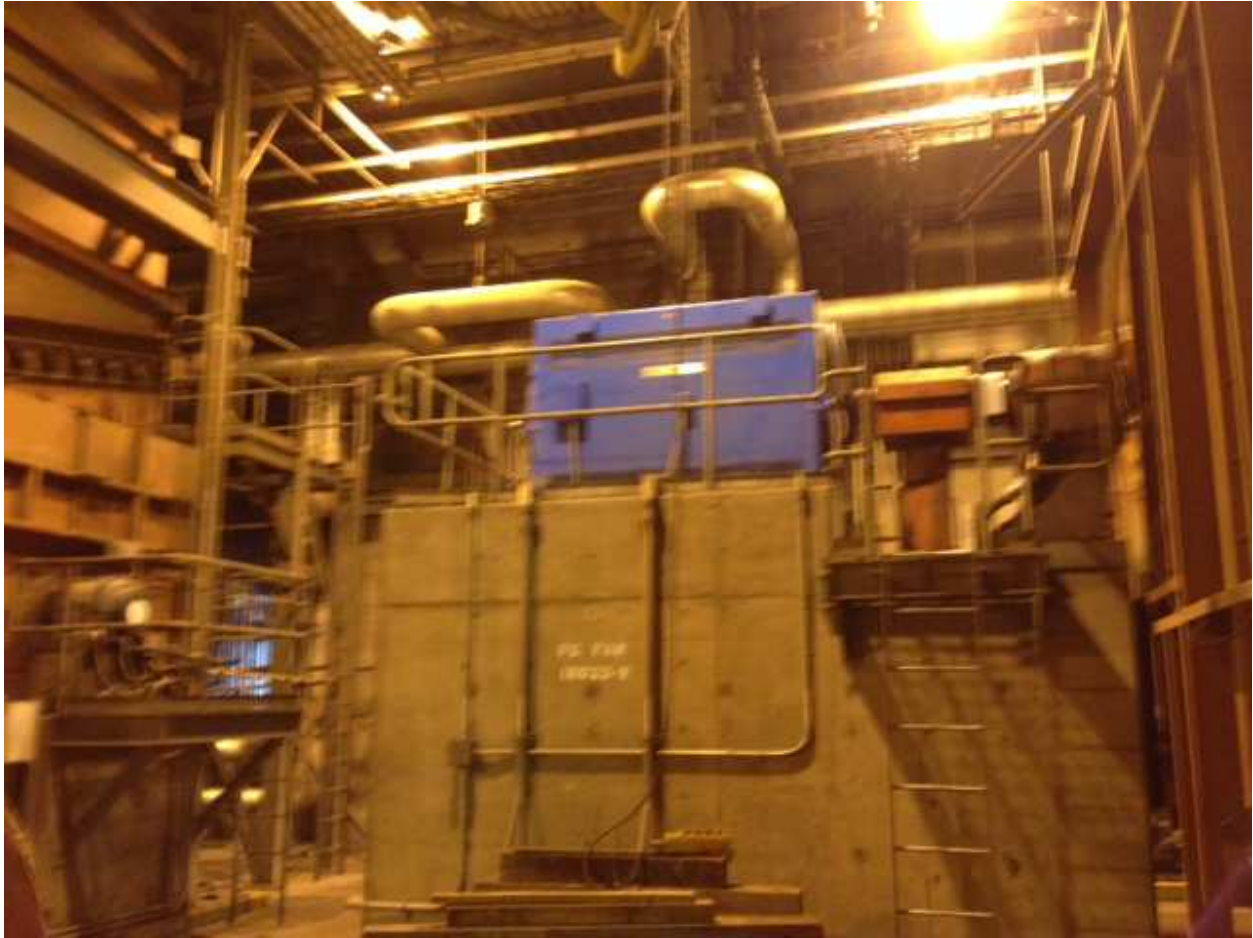
Forced draft fan motor on its pedestal
