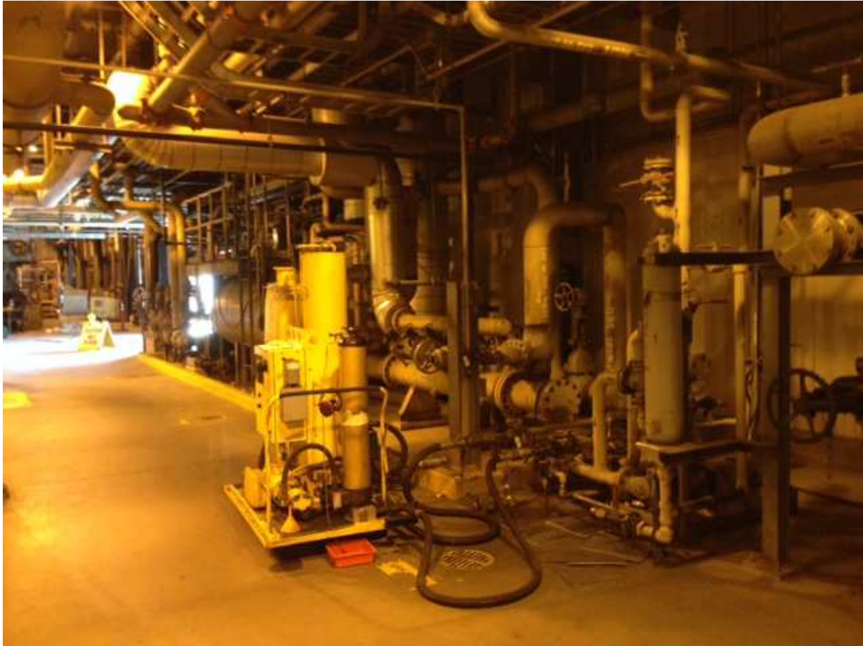
Turbine lube oil purification skid
