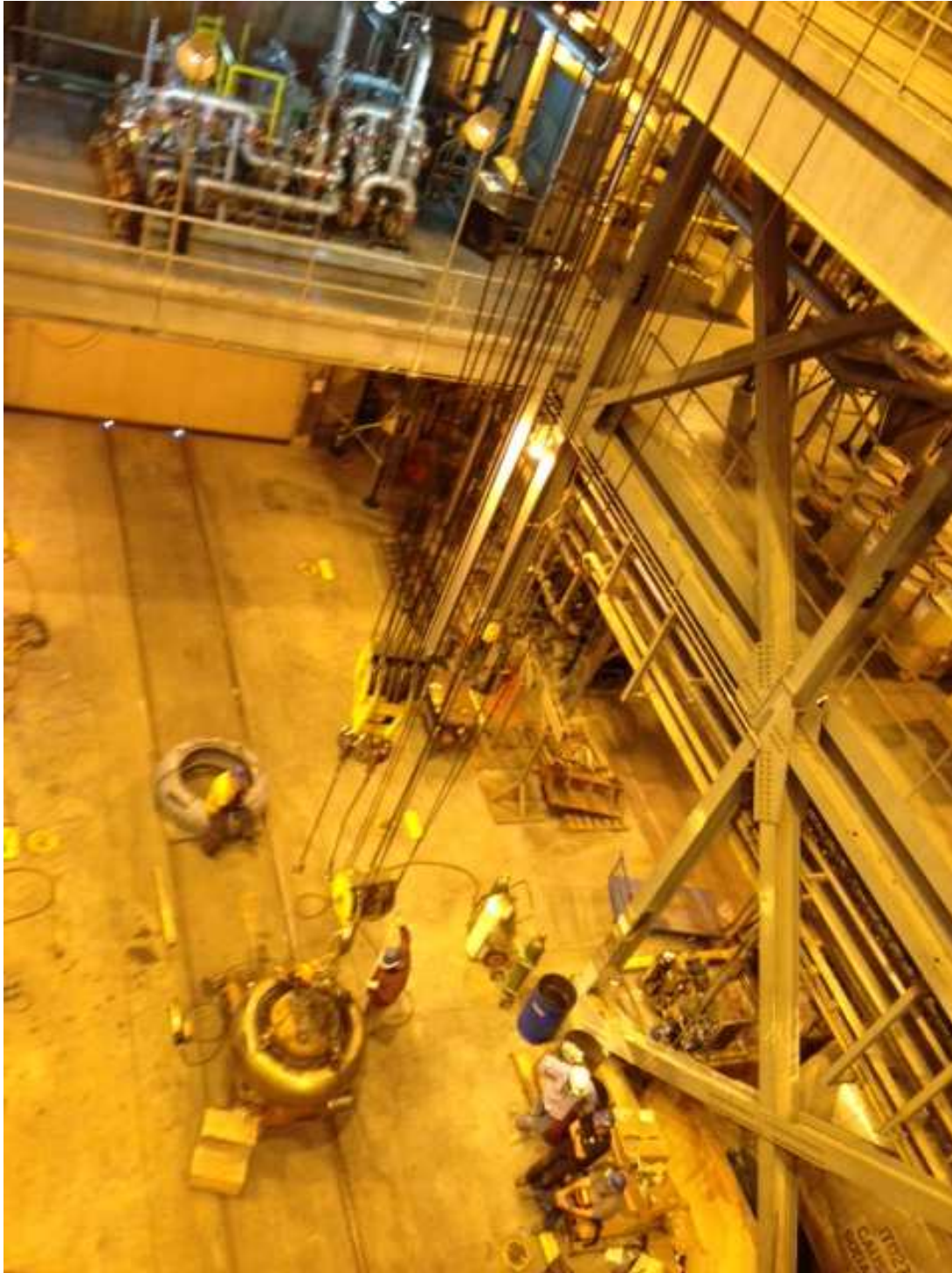
Looking down through the crane bay, pulverizer wheel repair on the ground floor, generator stator cooling water skid on the second floor
