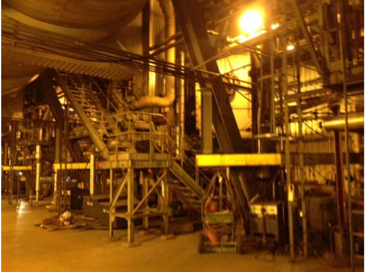
West Bottom Ash Hopper area
