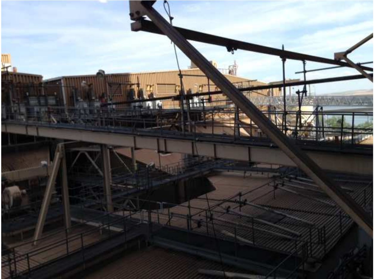
ESP access catwalk
