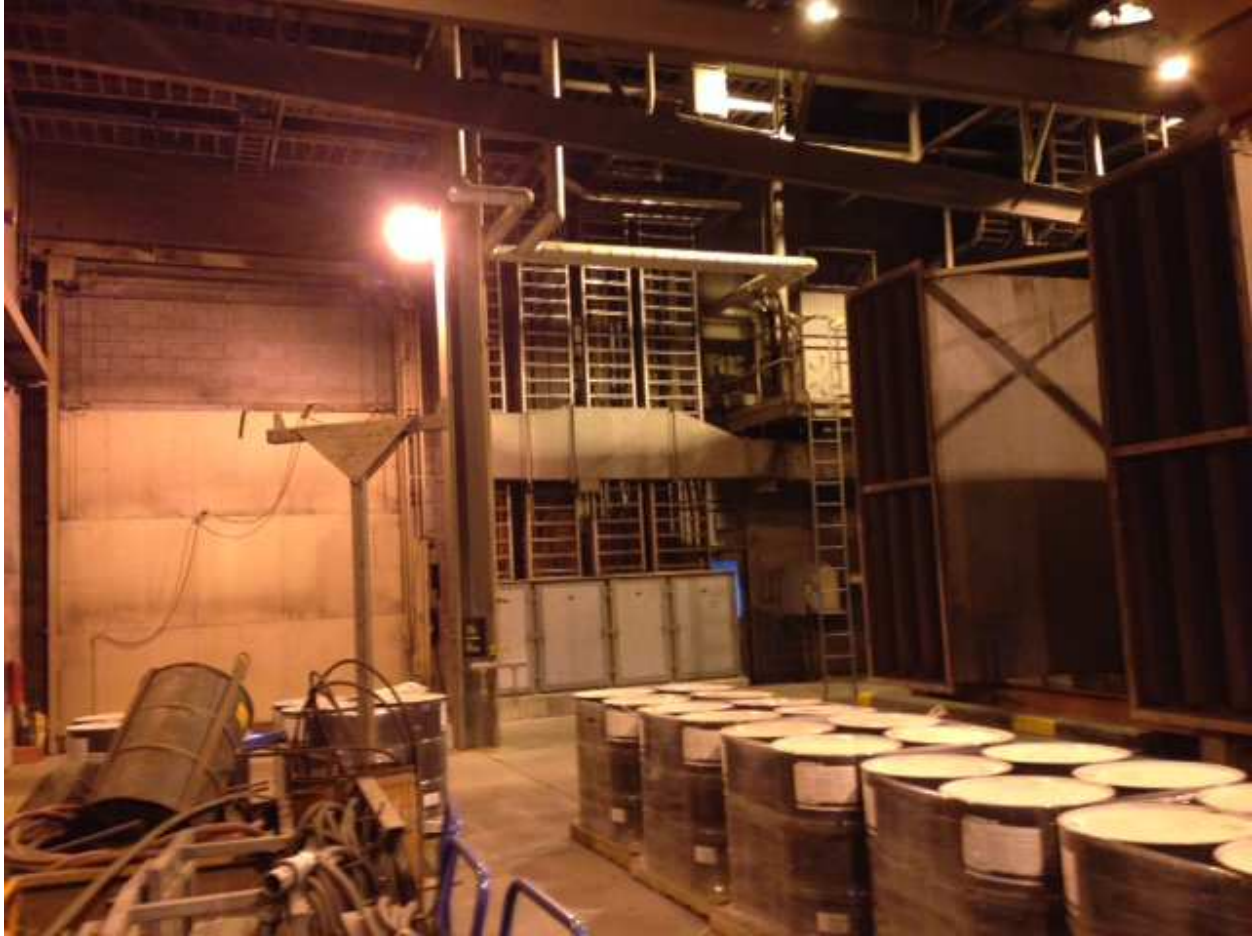
North fan room roll up door w/ barrels of Therminol 55 for the fan room air heating system
