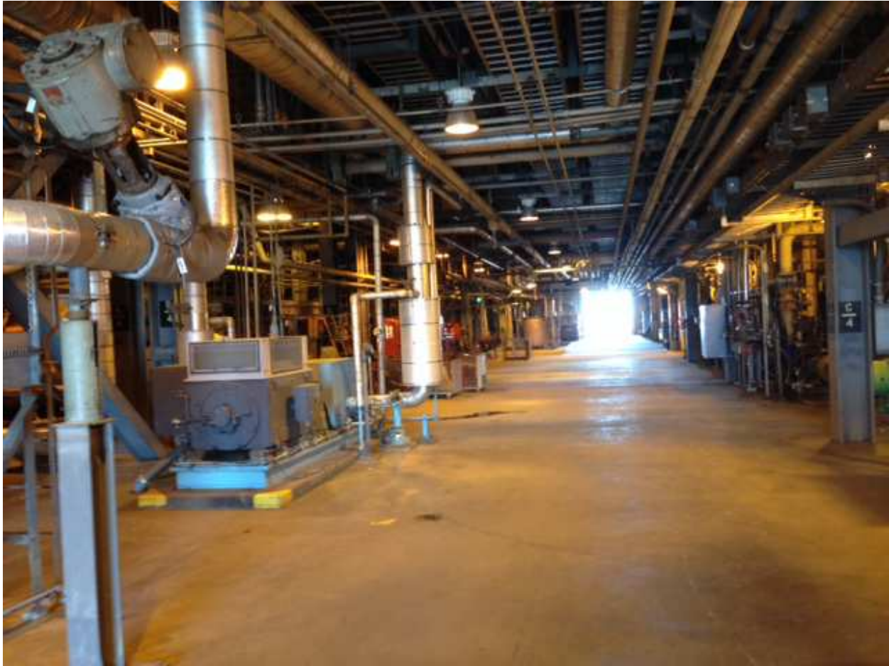
South view of Broadway, electric start up feed pump on the left
