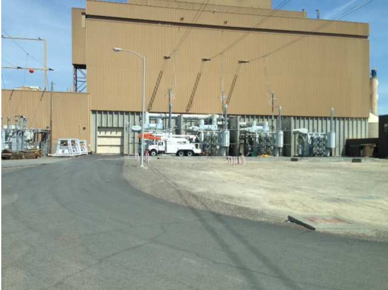
Main Transformers – west view of BCP
