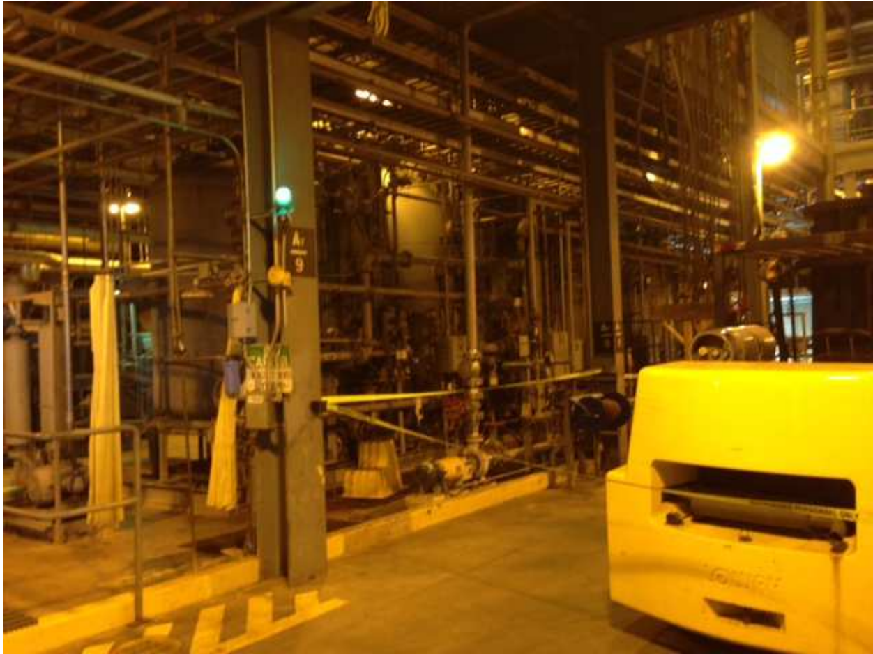
Condensate polisher system skid
