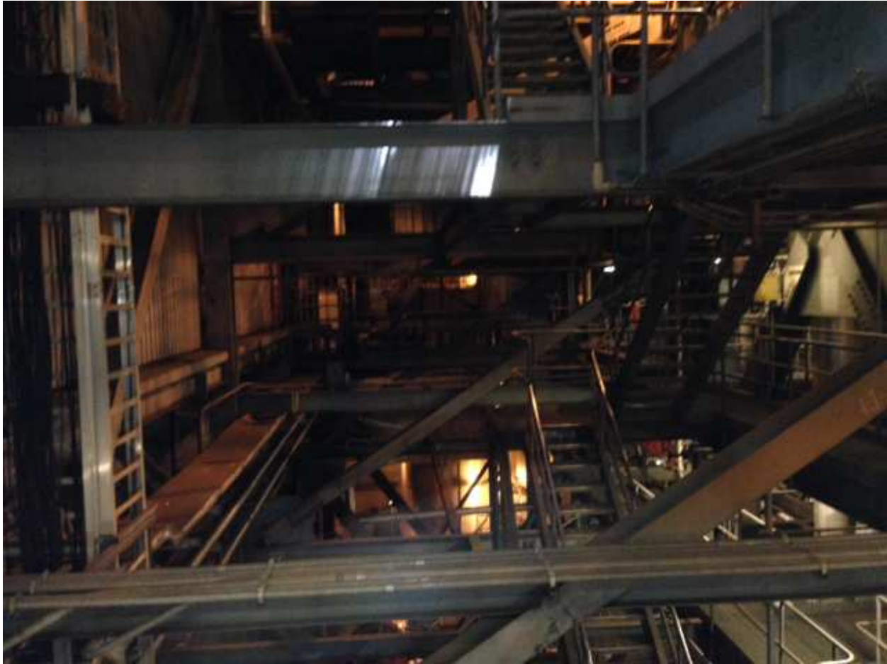
Coal gallery wall on the left, boiler on the right
