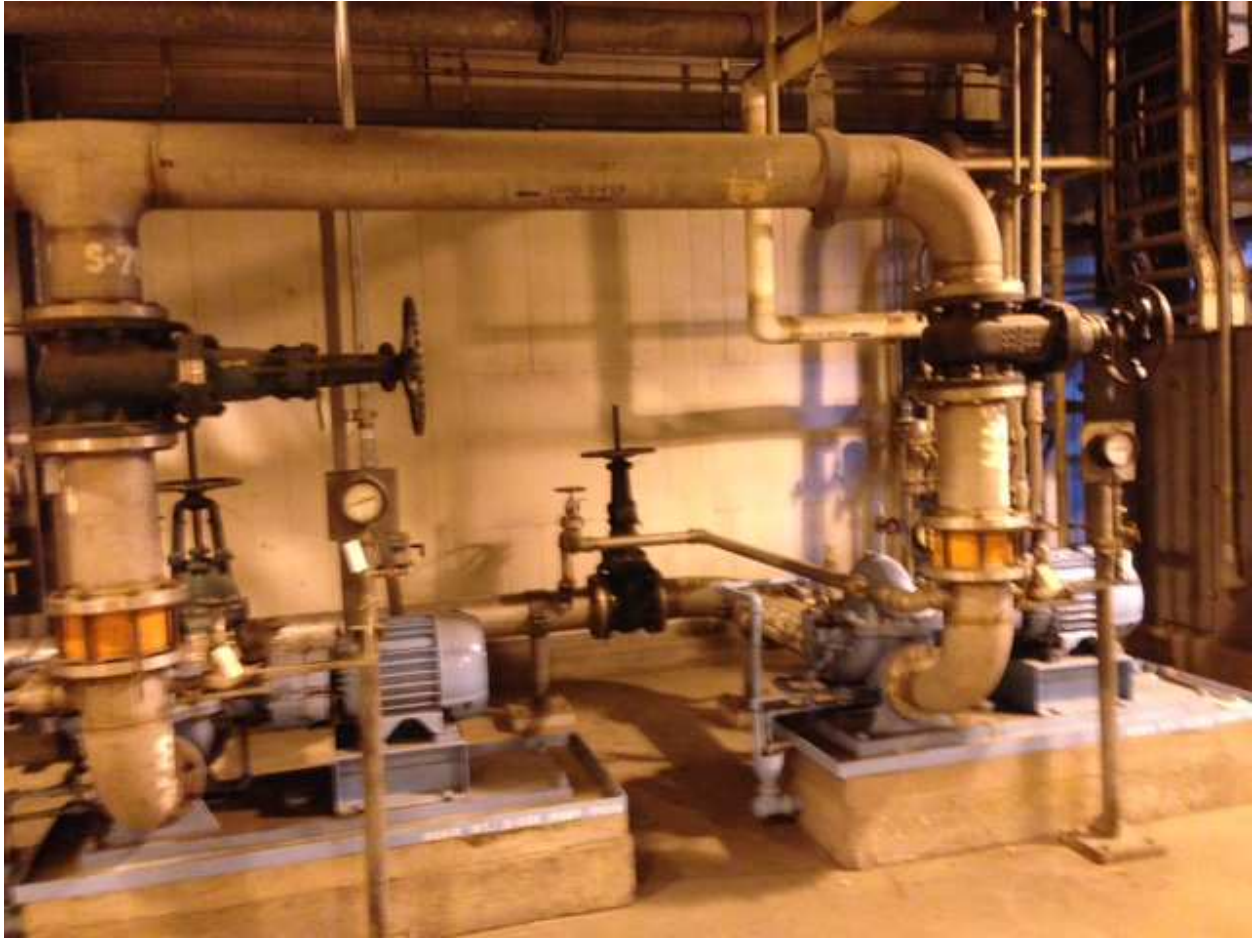
Condensate transfer pumps
