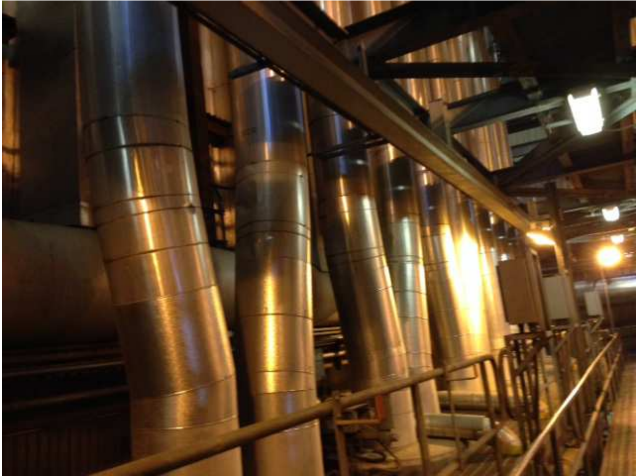
Downcomers from the steam drum to the bottom headers of the water walls
