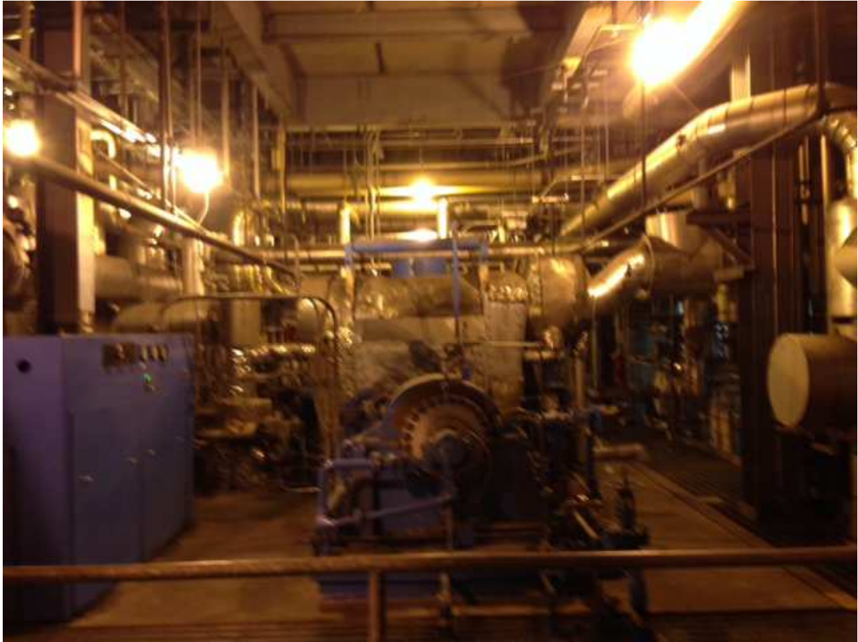
Feed pump turbine (FPT)
