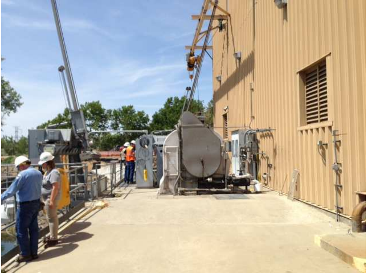
Service water travelling screen and trash rack rake
