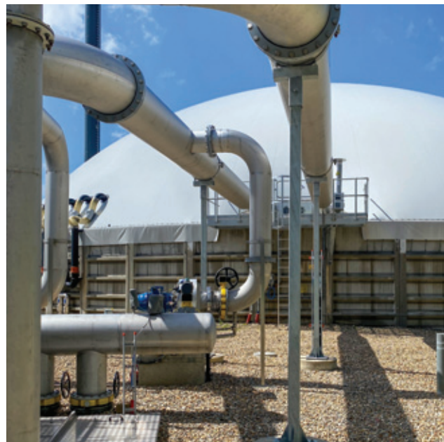
Gas process and storage equipment at the Nature Energy Korskro Biomethane Plant in Denmark.
