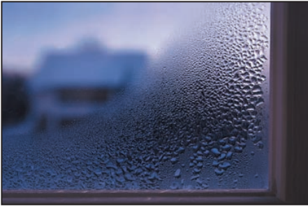
Condensation on the inside of a window-pane.
