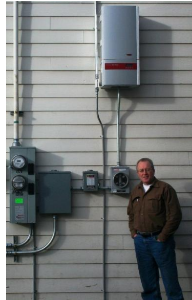
Figure 1: Dave Sullivan stands next to the electronics for his new solar system.
