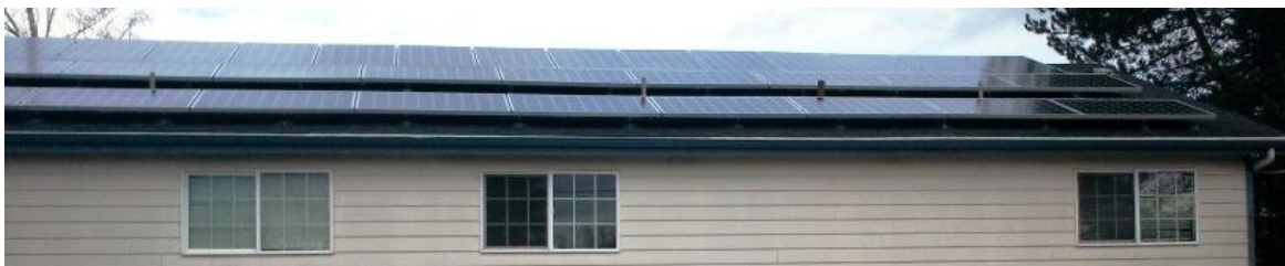
Figure 2: Sullivan's 9.4 kilowatt system almost completely covers the south-facing portion of the roof.
