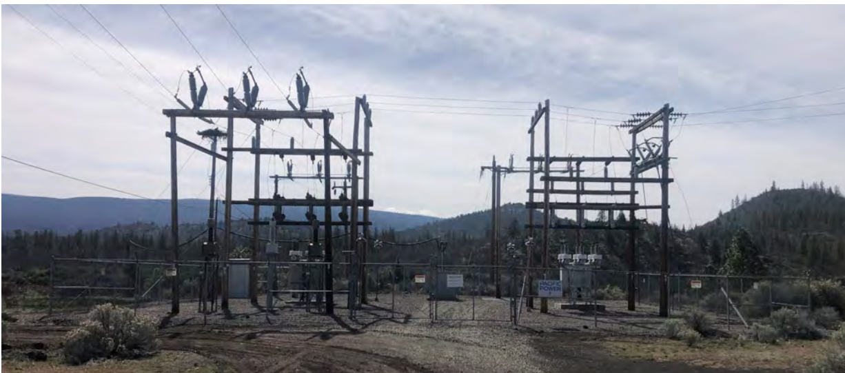
Photograph 5-1. Copco No. 1 Switchyard
