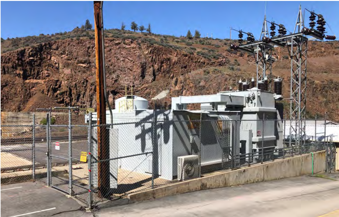
Photograph 6-1. Iron Gate Substation
