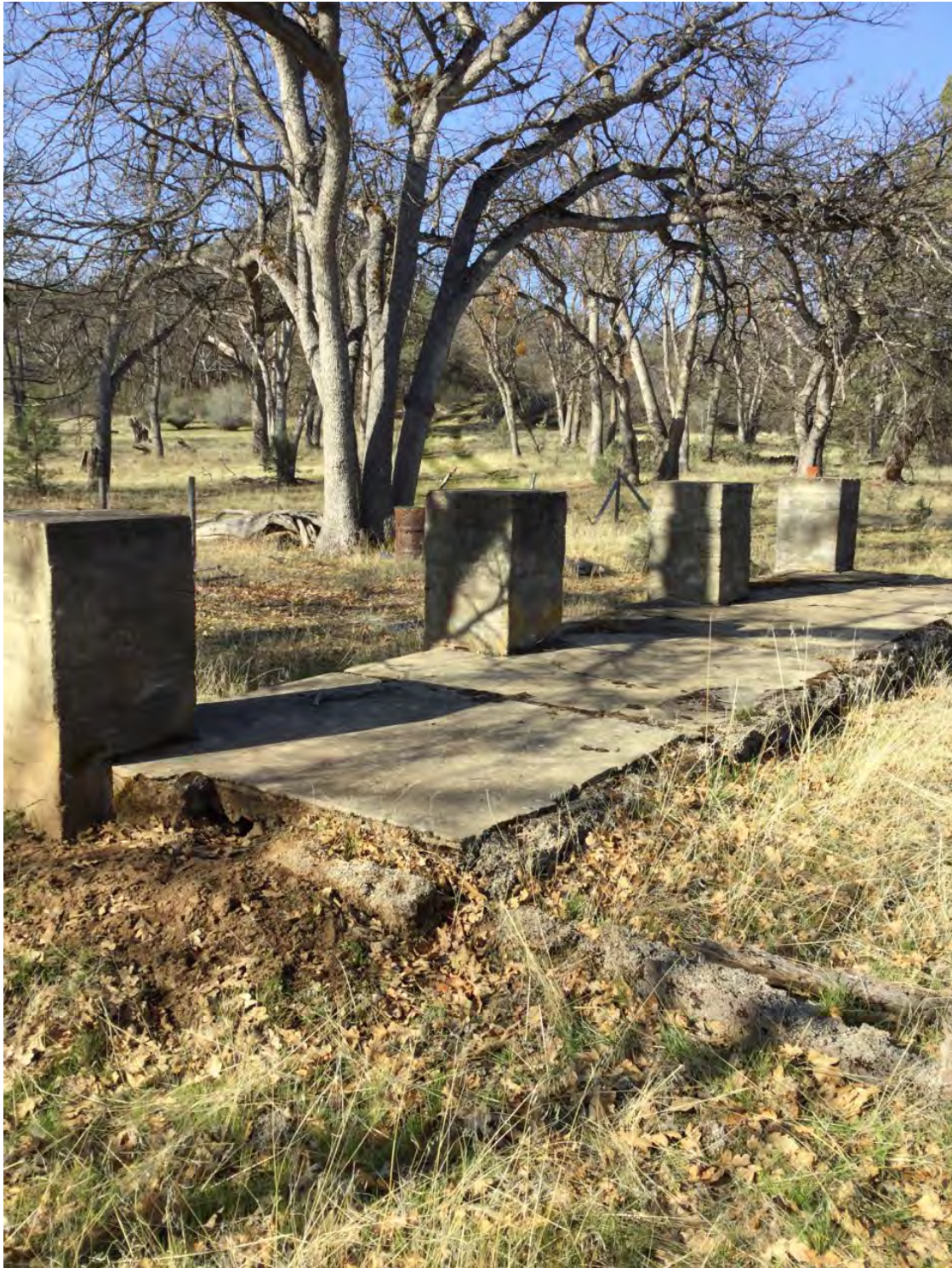
Photograph 15: Concrete – Old Foundation
