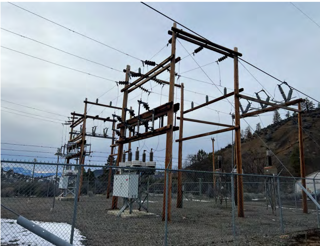
Photograph 5-2. Copco No. 1 Switchyard Transformers
