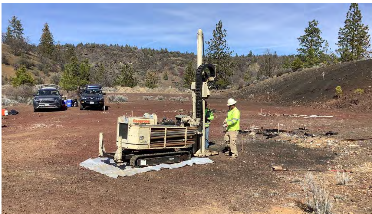
Photograph 5-2. Copco No. 1 Debris Pile/Scrap Yard Looking East at Area of Strewn Burned Material and Direct-push Technology Rig (Jacobs 2022a)
