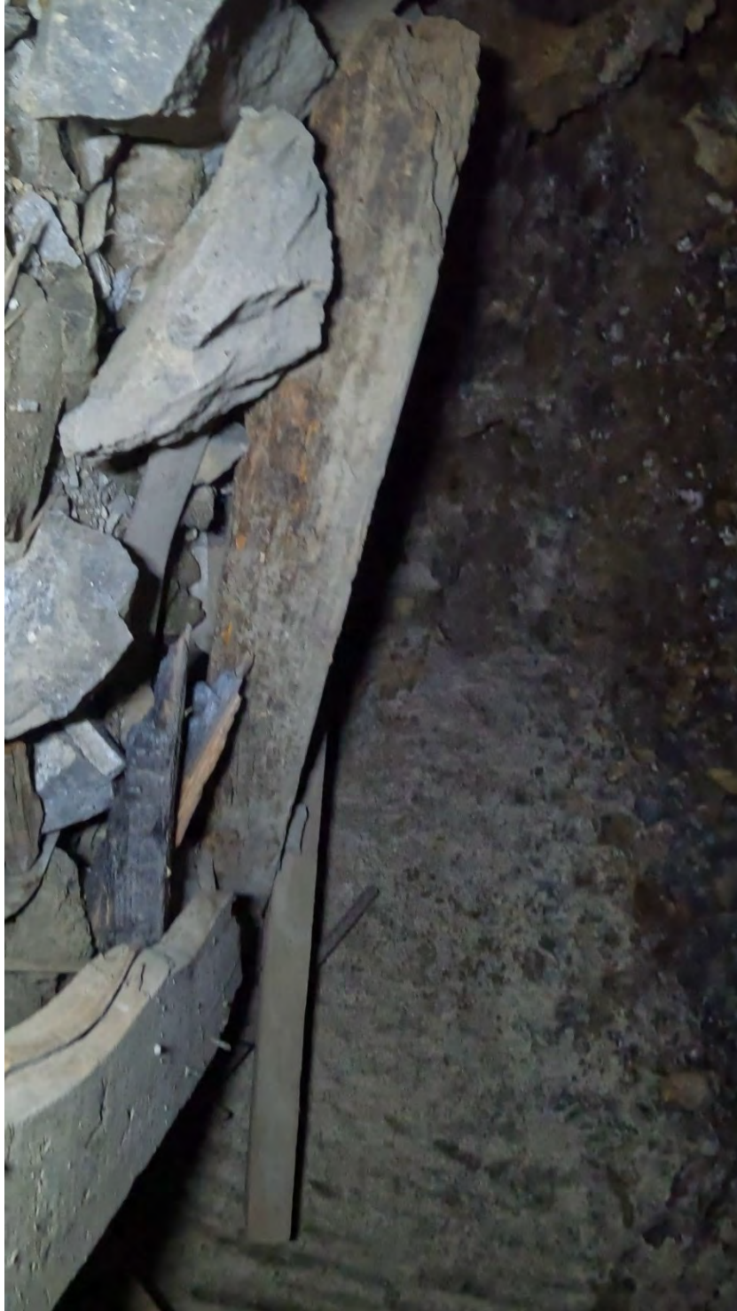
Photograph 10: Shaft Debris View 2
