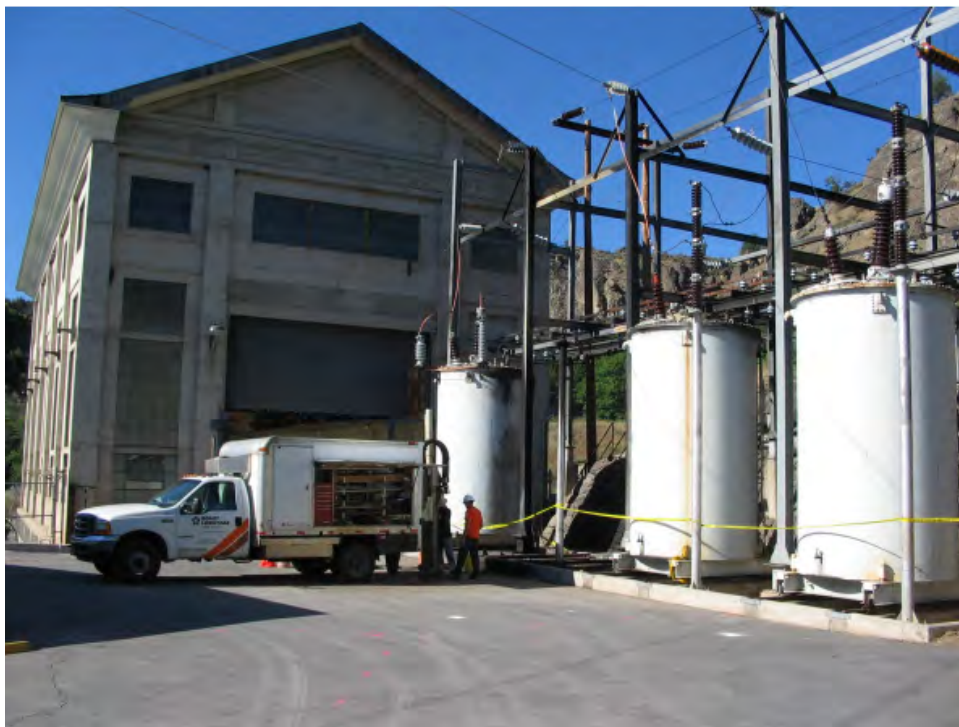
Photograph 3-7: Former Transformer C Location (removed) (Parametrix 2006)
