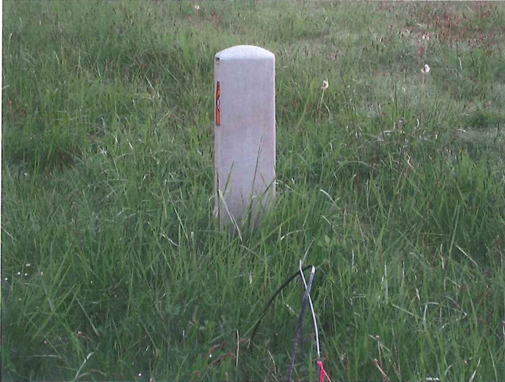
Probable violation 1a.: Temporary service comes out of pedestal and ground laid to a new home at 35536 Sunny Hill Lane, Pleasant Hill.
