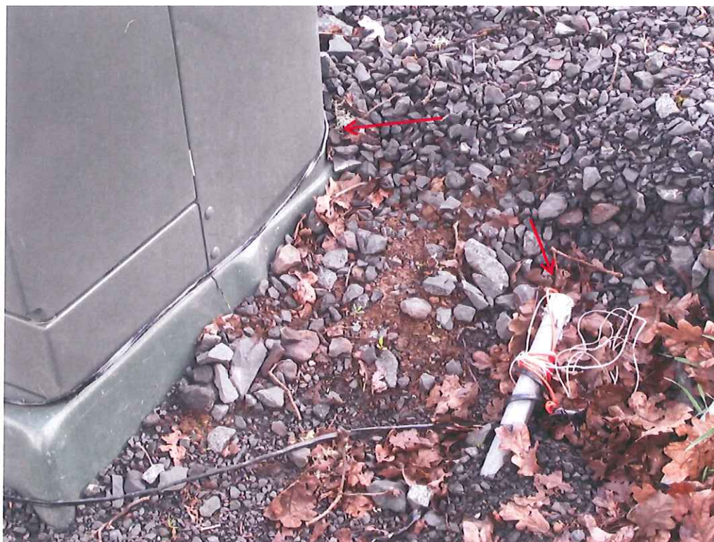
Cable is wrapped around a Emerald People's Utility District transformer. Then goes into a customer provided conduit next to the road, which comes up in their garage.
