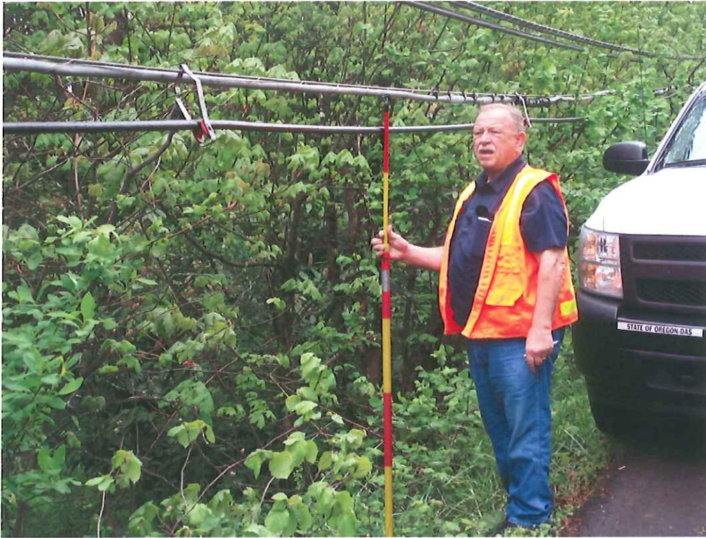
Cable has 6'2" clearance above edge of road between pole 1105/234340 and pole 1105/234441.
