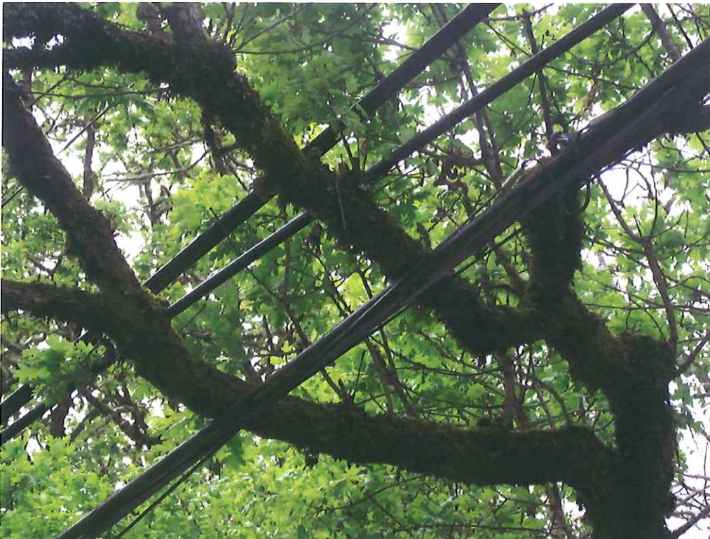
New temporary cable is laying hard on tree limbs in several locations.
