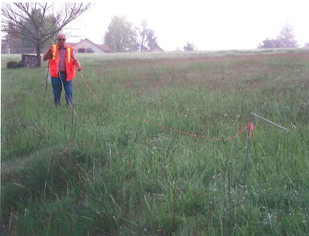
Cable is ground laid going south to a culvert approximately 110 feet.
