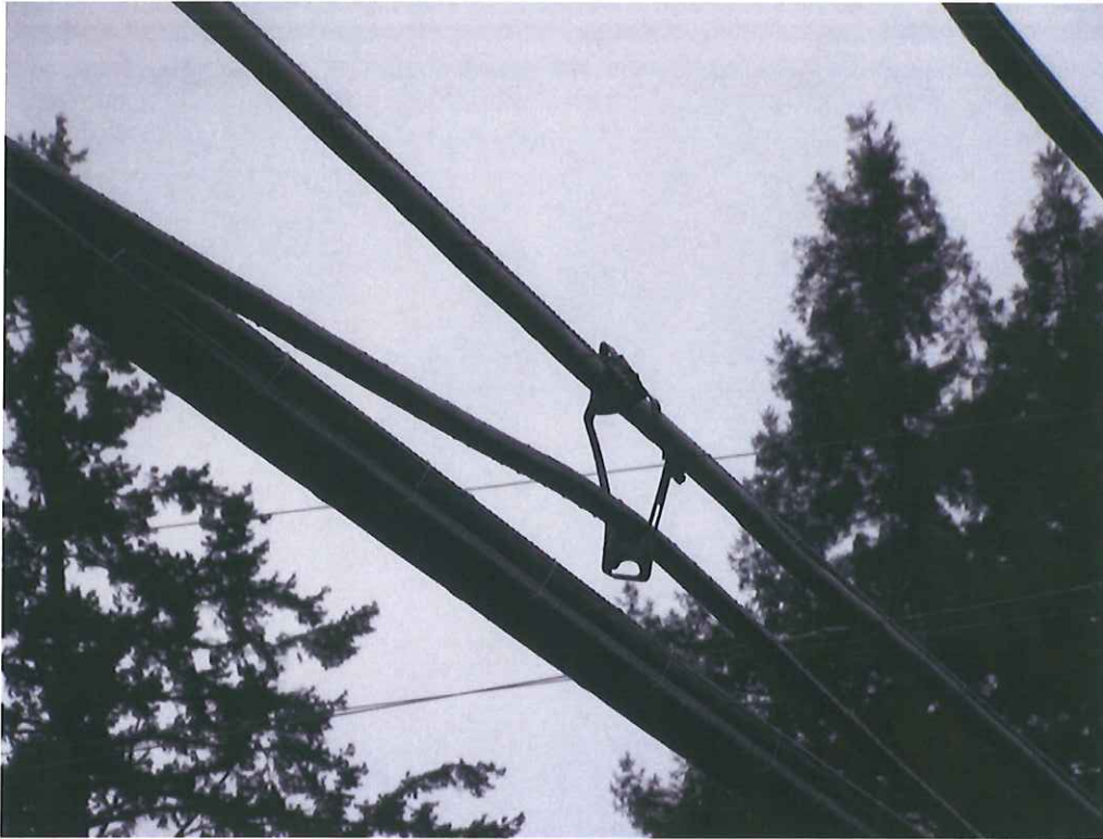
Cable was damaged in January 2014 and a new temporary cable was installed, which is supported in temporary rollers going north four spans to PacifiCorp pole 1105/234441.
