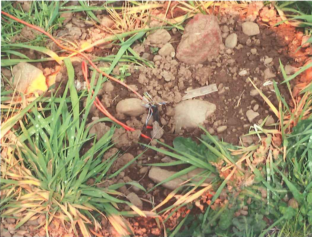
Probable violation 1a.: Temporary service to new home at 36849 Tovey Drive, Springfield is connected to a paired cable that's stub up out of street located at the NW corner of the intersection Sunderman Road and Tovey Drive.
