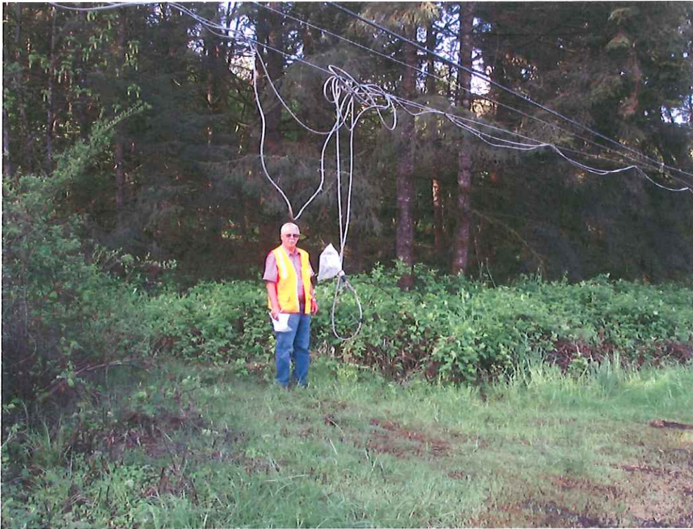
The cables and splice are hanging down near ground level.
