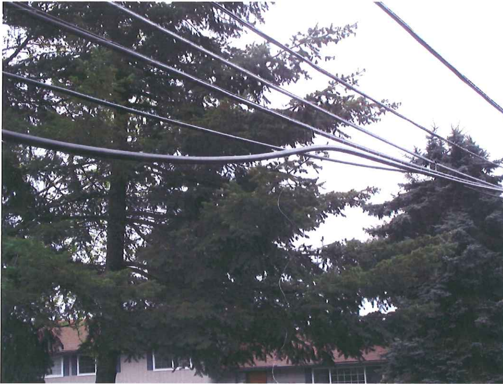
Probable violation 1a.: At the intersection of NW Highland Drive and NW Conifer Boulevard lashing wire is broken allowing cable to drop down to 9 feet above the ground.
