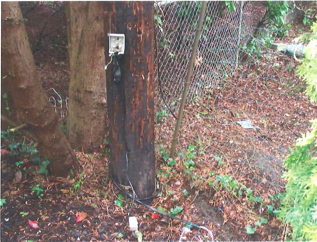
Probable violation 1a.: Behind 2650 Roosevelt Drive, CenturyLink dropped a cable from the aerial wire down PacifiCorp pole 01311005/275906, CenturyLink # 2656/R, and wrapped it around base of pole.
