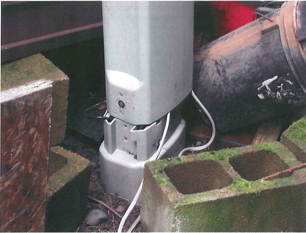
Probable violation 1a.: Two communication cables comes out of pedestal behind carport for space 100 in Heatherdale Mobile Home Park
