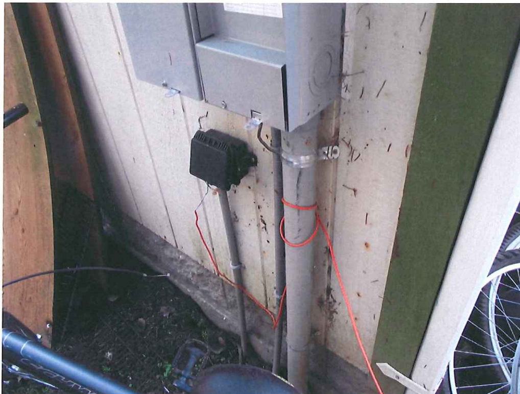
Cable is wrapped around the meter base conduit before terminating in subscriber network interface on shed.
