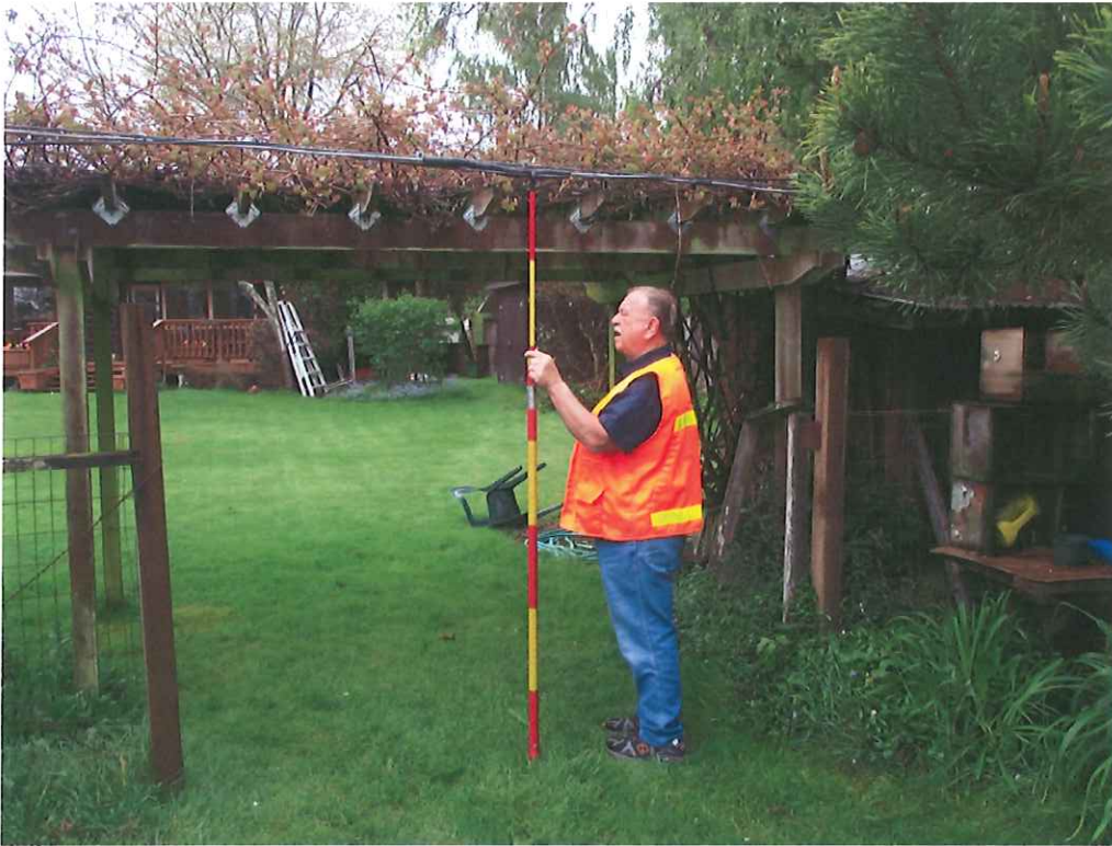
Probable violation 1a.: Communication cable has 7'1" clearance above the ground, creating a hazard at 3700 Jackson Street, Corvallis.
