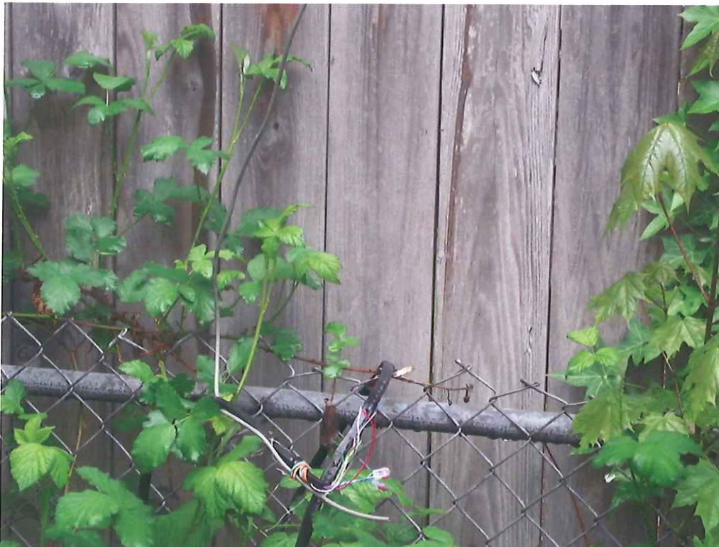
Cable is spliced into cable going up PacifiCorp pole 1105/275943, CenturyLink # 2650 R, and attaches to cable serving 2315 27th Street.
