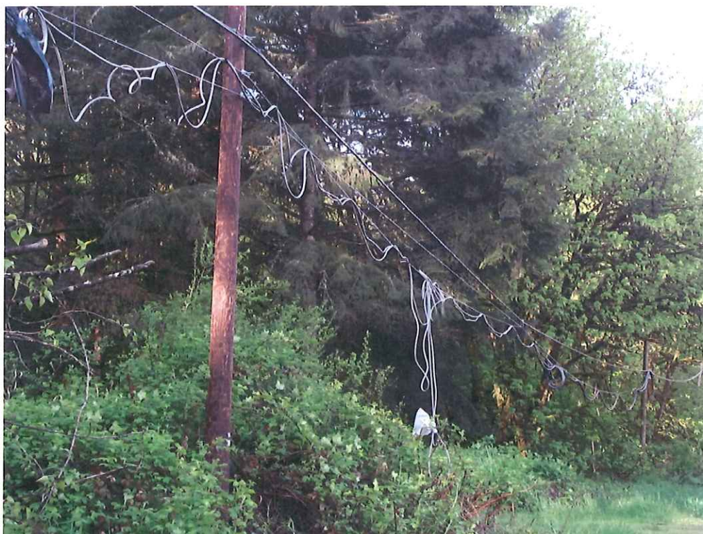
Approximately 100 feet of 2 main cables have been temporized with another cable.
