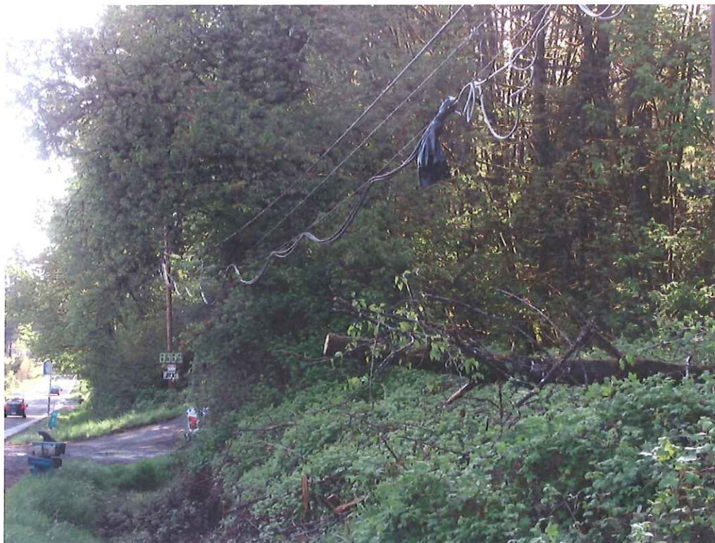
Probable violation 1a.: Tree fell into line breaking off pole and damaging two communications cables during snow storms in early February. Located in the two spans west of 8385 McKenzie Highway, Springfield.
