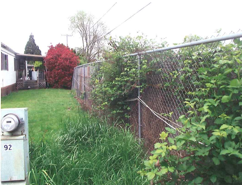
Two cables are either ground laid or tied off to fence going approximately 100 feet east, located on the north side of mobile home in space 100.
