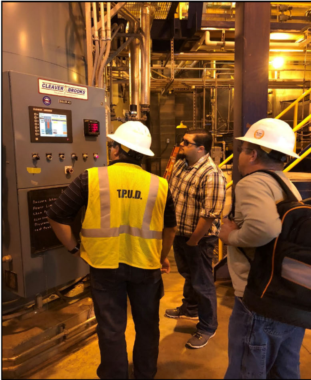
Cleaver Brooks 5 MW Electric Boiler - Derek Mickelson and Glenn Johnston on site with TCCA engineering staff to ensure the breaker relay would coordinate properly with the PUD switch gear that provides service to the boiler.
