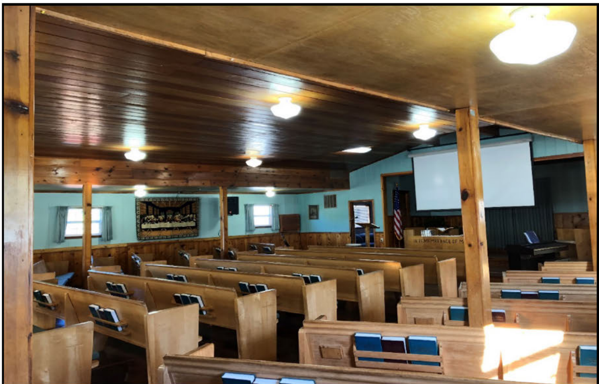
Chapel Hall Interior – Retrofitted the 75 watt “school house” fixtures to 10 watt LED.
