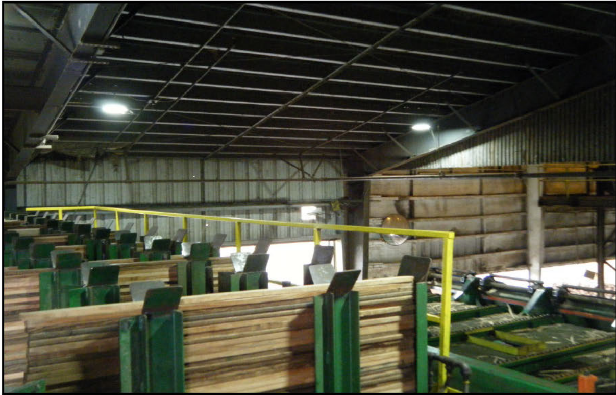
Saw Mill #2 Stacker – 150 watt LED fixtures installed.
