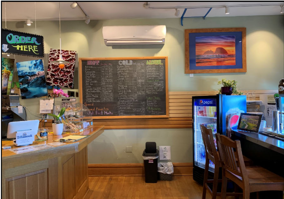
3-Ton Ductless Heat Pump Installed.
