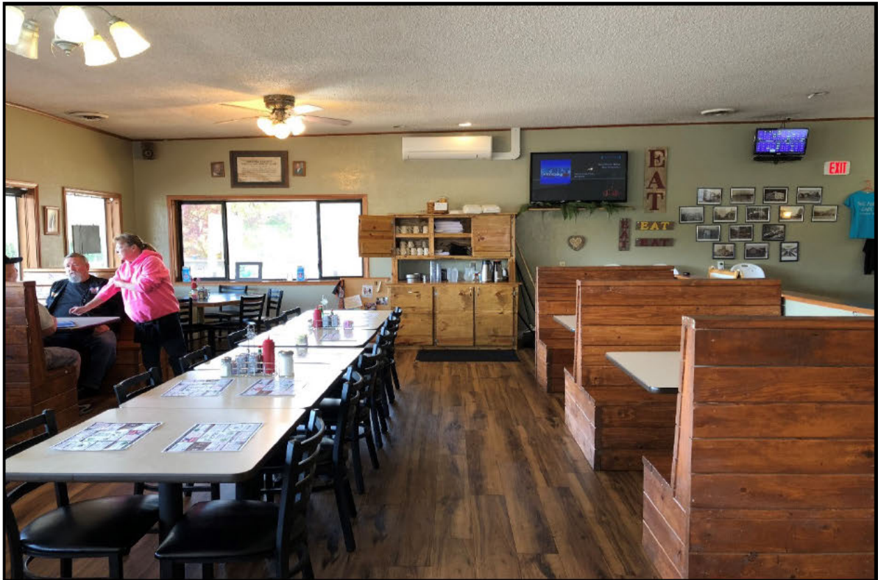
The Fern Restaurant – Ductless Heat Pumps Installed.
