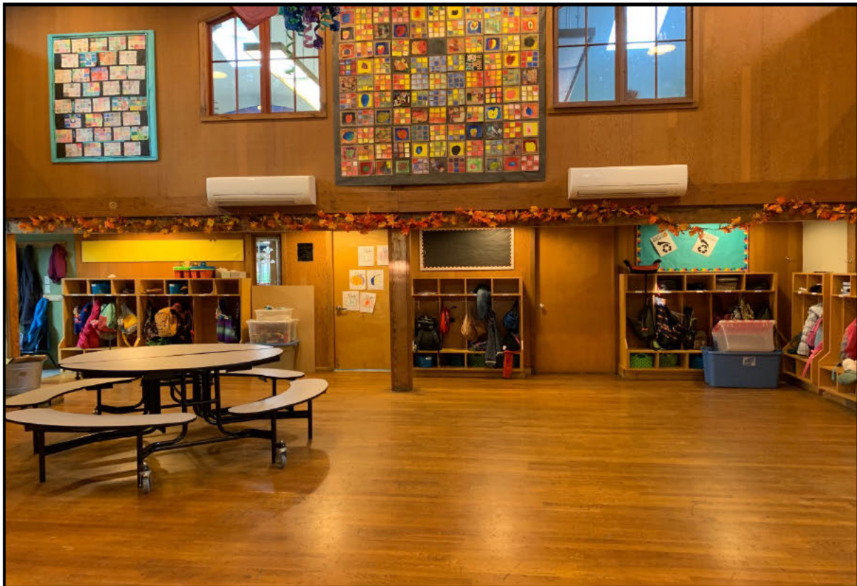
2-Ton Ductless Heat Pumps Installed.
