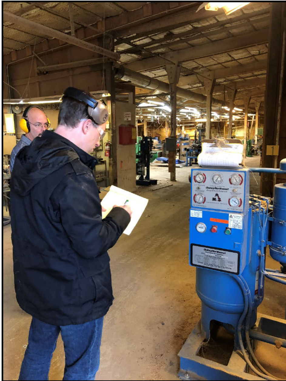
Jimmy Sauter – Recording the operating pressure and air flow on the 50 HP Quincy single speed air compressor.
