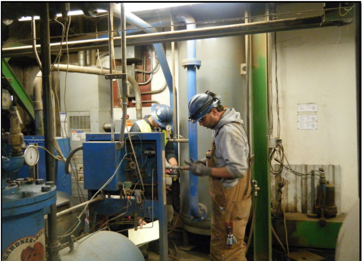
Stimson Lumber Staff – Installing an air fitting and air-flow data logger on the main air supply line from the compressor room to the mill.
