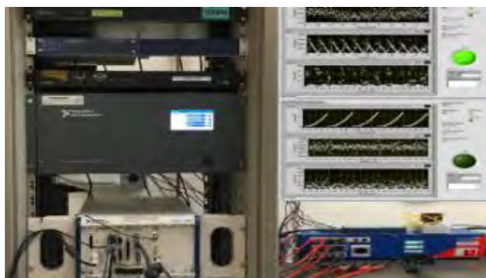
Figure 2. Calibration Lab Implementation
