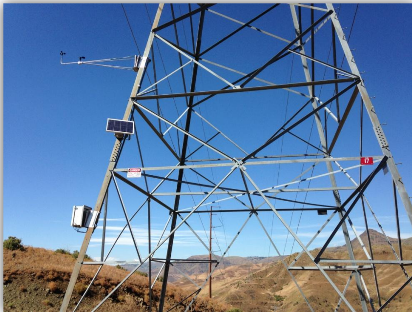
Figure 2. Dynamic Line Rating Equipment Installed in Hells Canyon
