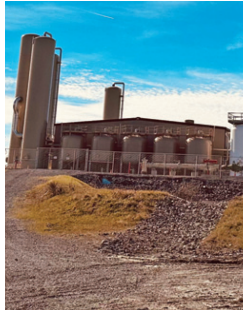
Limestone RNG Facility that NW Natural Renewables is investing in.
