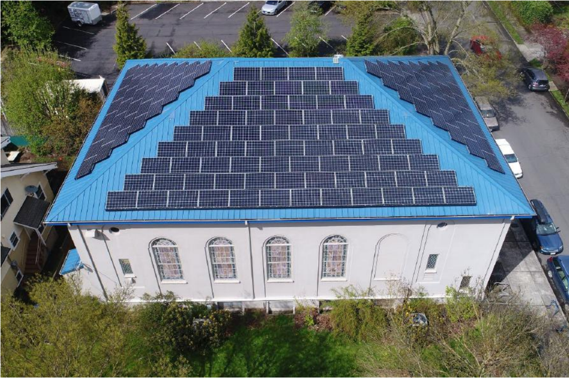
39.6kW Grid-Tied Solar PV System Mazama Mountaineering Center | Portland, Oregon
