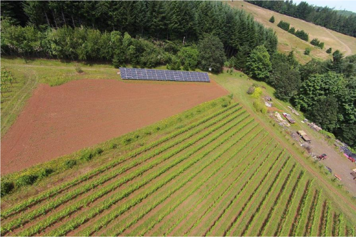
31kW Ground-mount Solar PV System Log Homes Store + Vineyard | Sheridan, Oregon
