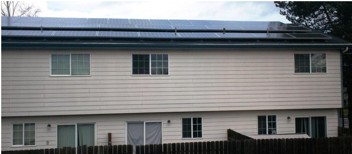
Figure 1: Solar panels on the roof of Dave Sullivan’s four-plex in Albany.
