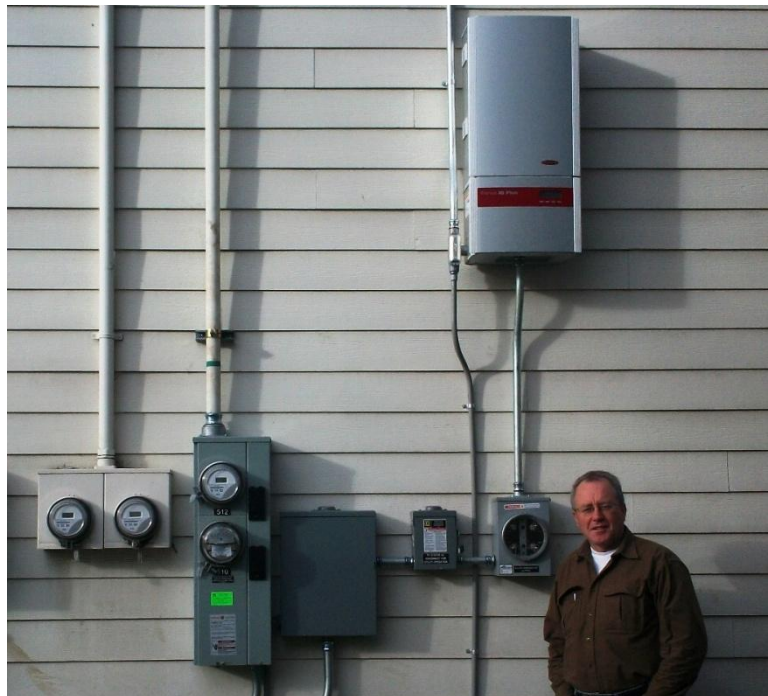
Figure 3: Dave Sullivan stands next to the electrical equipment for his new solar system.
