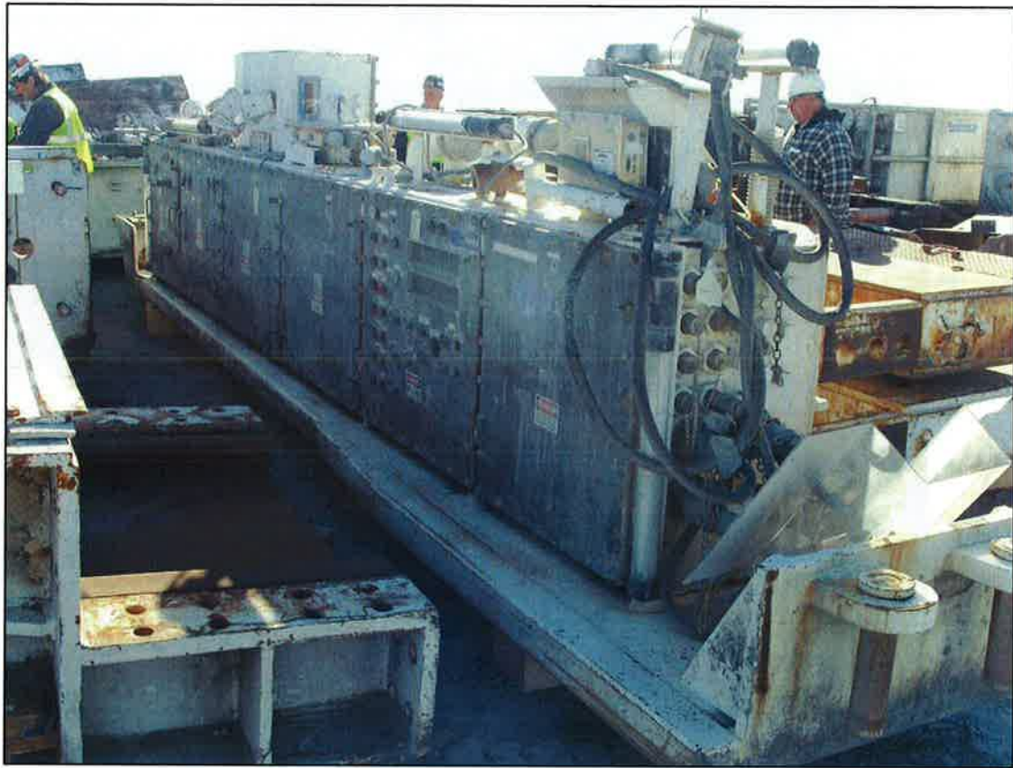
Master Control Station, 22-218
