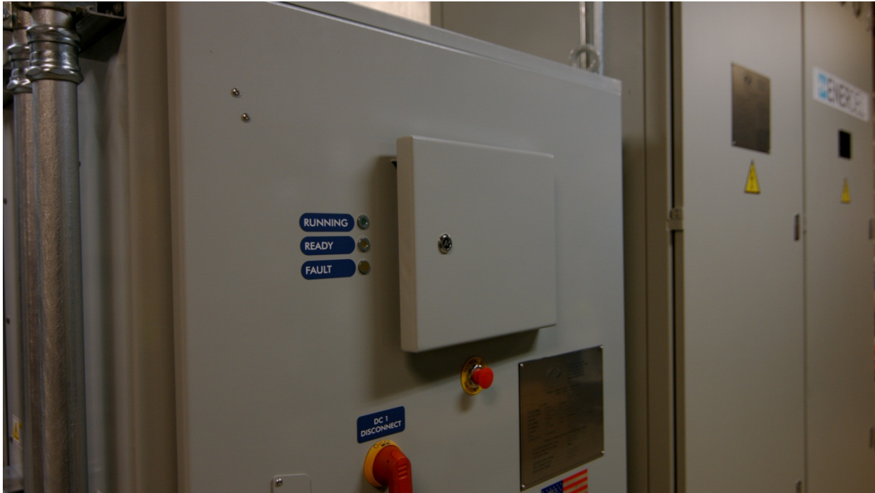
Figure 3-3 Lithium Ion Battery Energy Storage System Located at Black & Veatch HQ
