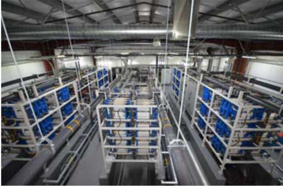
Figure 5-4 Vanadium Redox Flow Battery (Source: Prudent Energy brochure)
