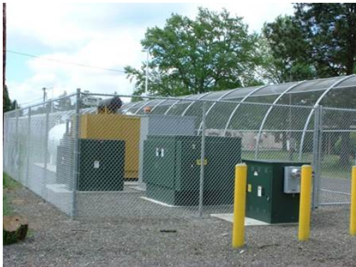
FIGURE 7-5: Generator at MacLaren Youth Correctional Facility
