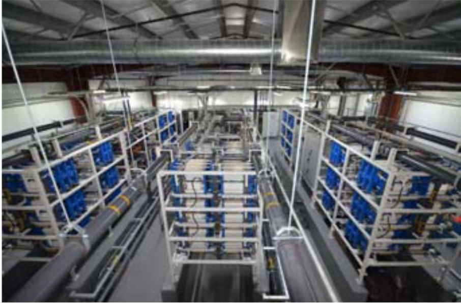
Figure 3-5 Vanadium Redox Flow Battery (Source: Prudent Energy brochure)
