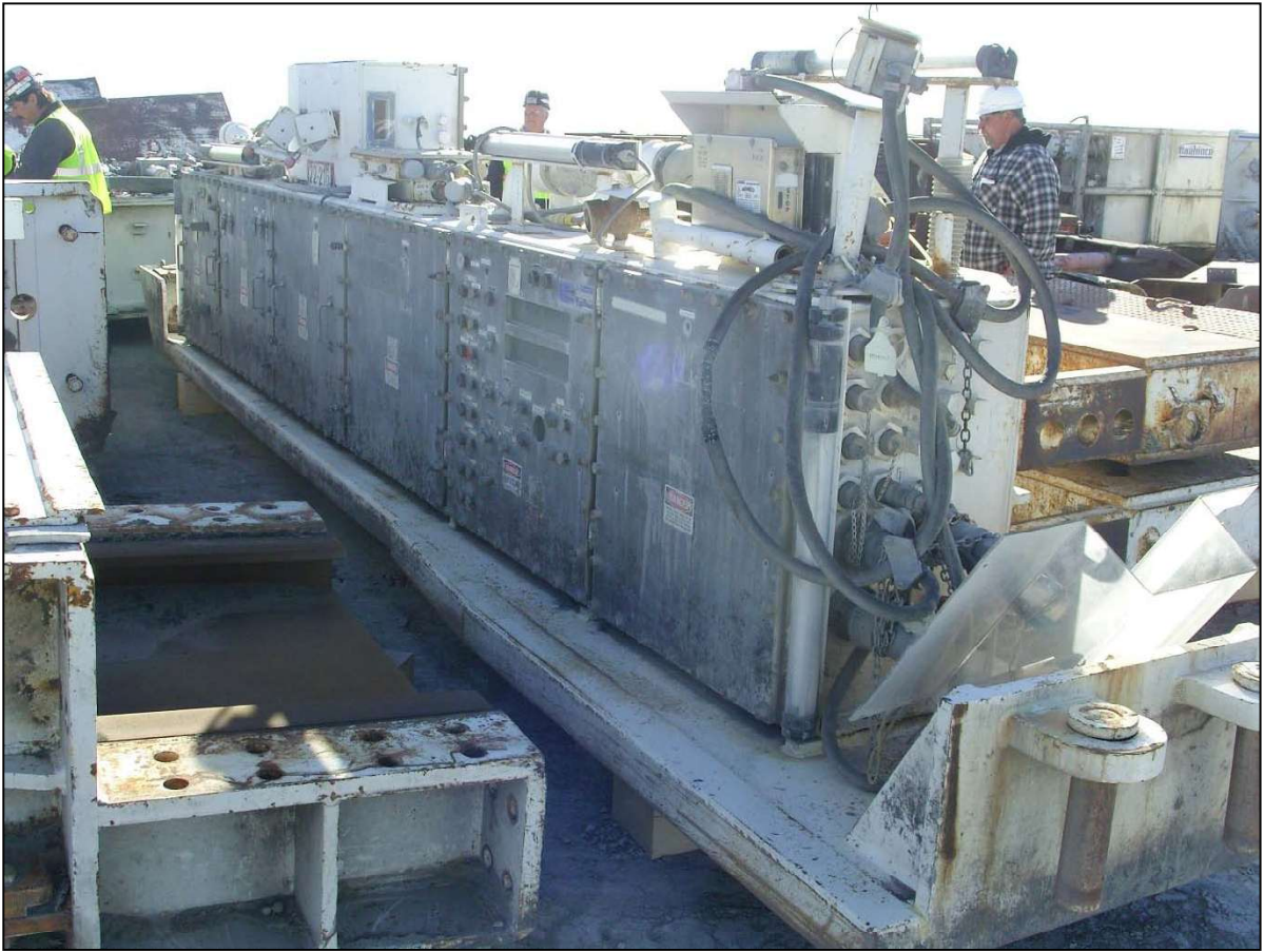
Master Control Station, 22-218
